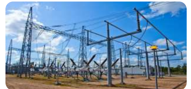
Utility substations: Balance of System, battery charging, power to critical loads
