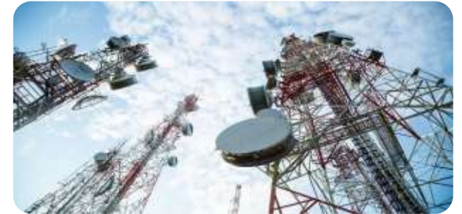
Telecommunications: remote towers, OPEX reduction of DG
