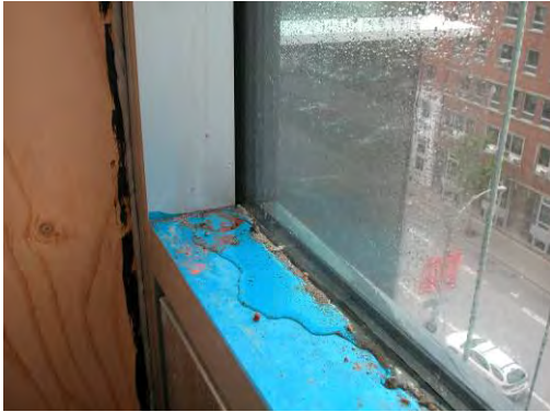
Figure 5: Example of water infiltration within a curtain wall assembly.
