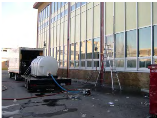
Figure 33: Portable water reservoir and pump system.
