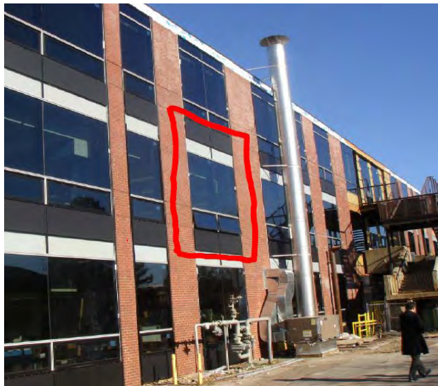
Figure 18: Identification of representative area for field testing (metal and glass curtain wall and adjacent masonry assembly).
