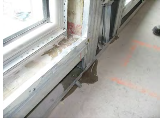
Figure 6: Example of water infiltration at a punch window assembly.
