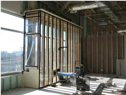
Figure 20: Interior test chamber used to test a portion of curtain wall section.
