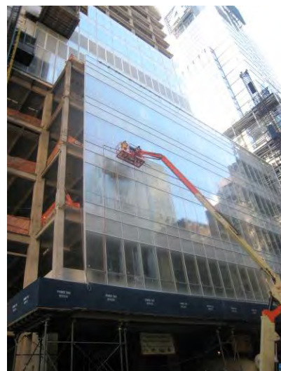
Figure 32: Calibrated sprinkler rack hung from motorized man lift.
