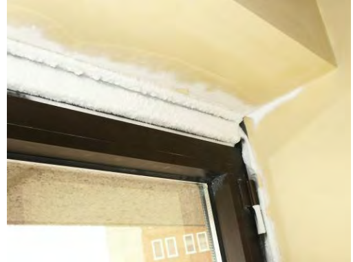
Figure 8: Example of excessive interior frost formation due to excessive air infiltration at a window/wall interface.
