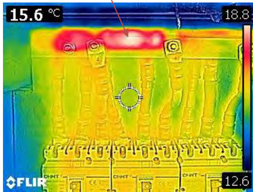
Hot spot in LV distribution box
