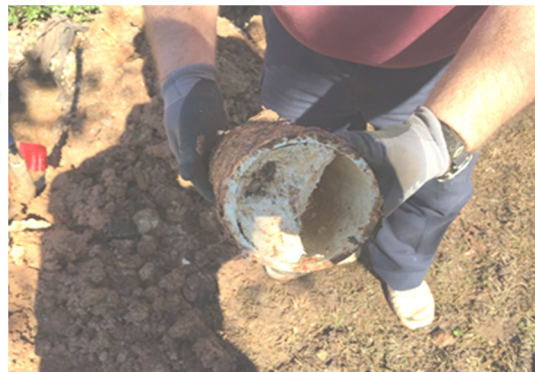
Hard grease in Mr. Jackson’s pipe
