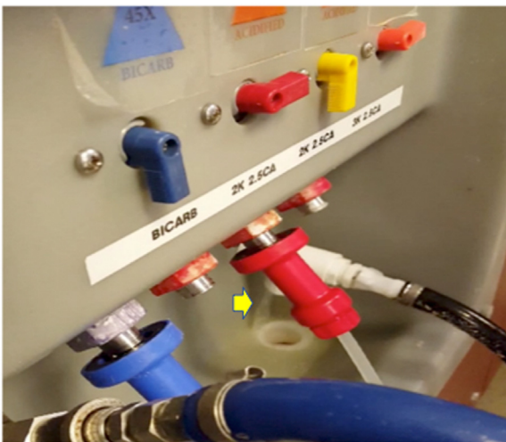
Fig 3. Wall box with white spigot and drain on right side of wall box. In the air space between spigot and drain, spent dialysate can be seen splashing into wall box next to the drain (arrow). (Figure is 1.5 or 2-column fitting image. Should be printed in color in print.)
