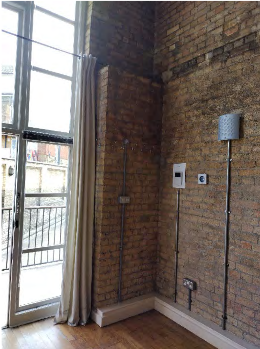
Figure 4: corner of the building with a brick pillar and marks on the wall which seems suggesting the presence of a mezzanine level.
