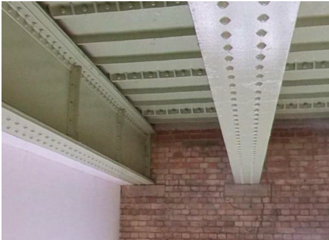
Figure 3 The giant "I" beams supporting the roof and the water tank above it.
