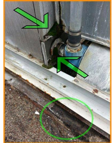
Leaks and Damage
