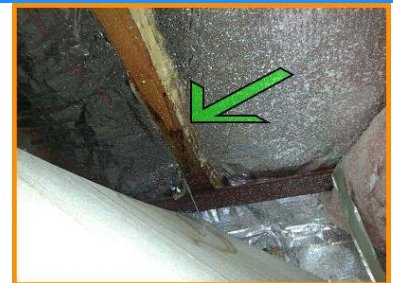
Stains - Framing and Drop Ceiling
