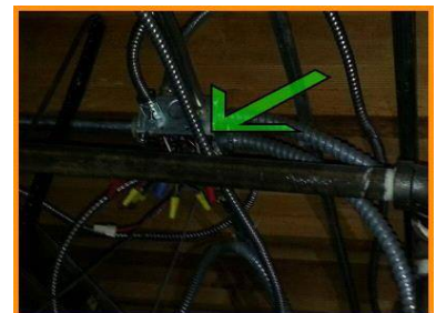
Box too small for # wires?
