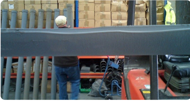
Examples of poor quality, warped gutters
