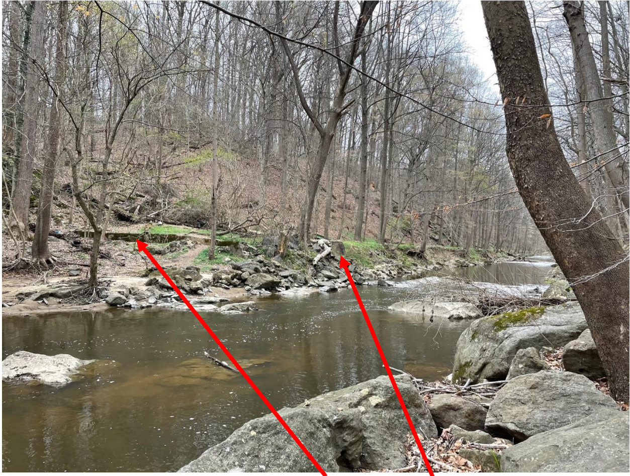
Looking upstream, the remains of the “Small Dam” and manhole structure next to it
