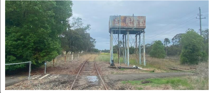
Figure 7 Heritage water tower at Weston, with the platform behind. The site has easy access from Station Street (foreground) and the remnant of the former second track is visible to the right.
