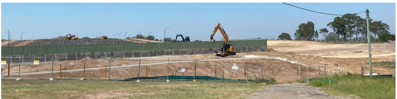
Figure 15 Housing development works underway at Gillieston Heights, December 2023. This photo was taken near the potential station site; the rail line is on the right.
