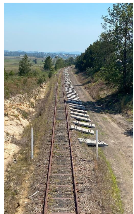
Figure 18 Rail corridor looking north from Kiah Road towards Maitland. The former location of the second track is evident.
