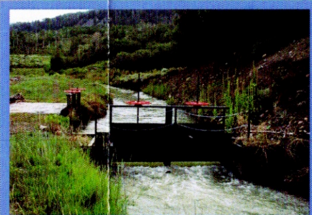
A typical headgate along the canal, which controls the flow and distribution of water to users.
