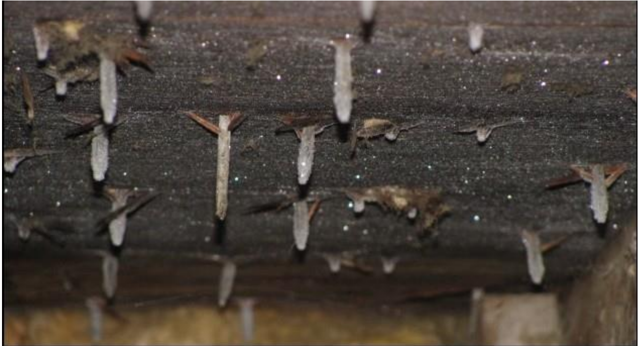
Attic Ceiling Mold With Frosted Nail Heads in the Winter
