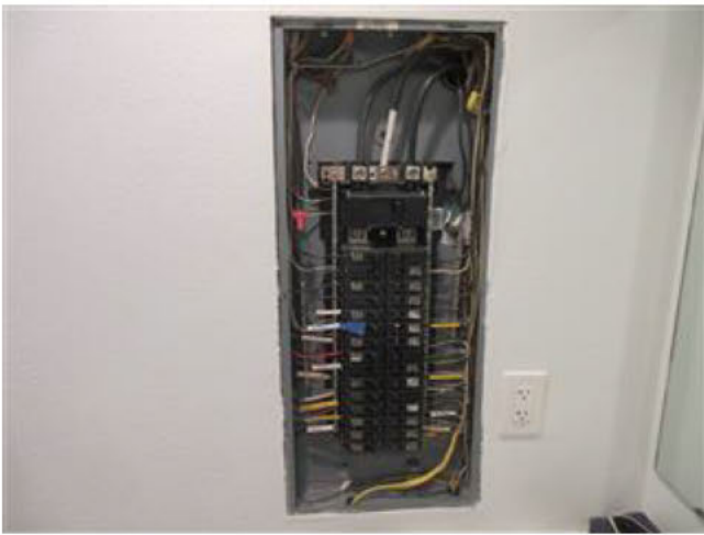
Main Panel Cover Off
