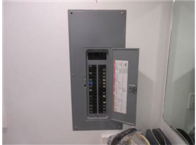
Main Panel Cover On
