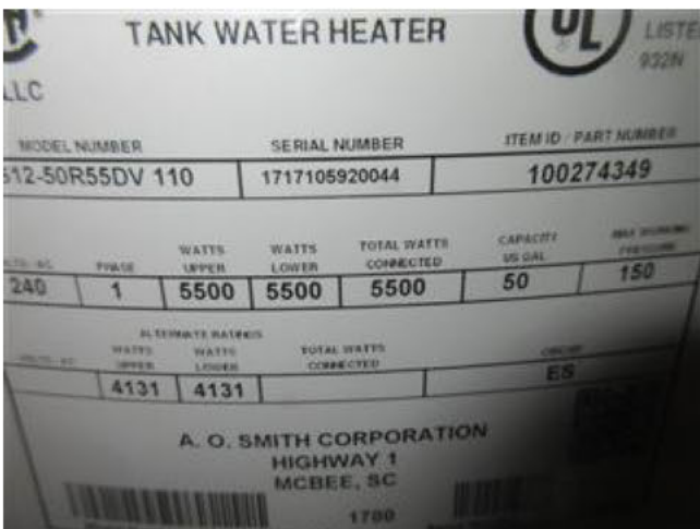
Water Heater Data Plate
