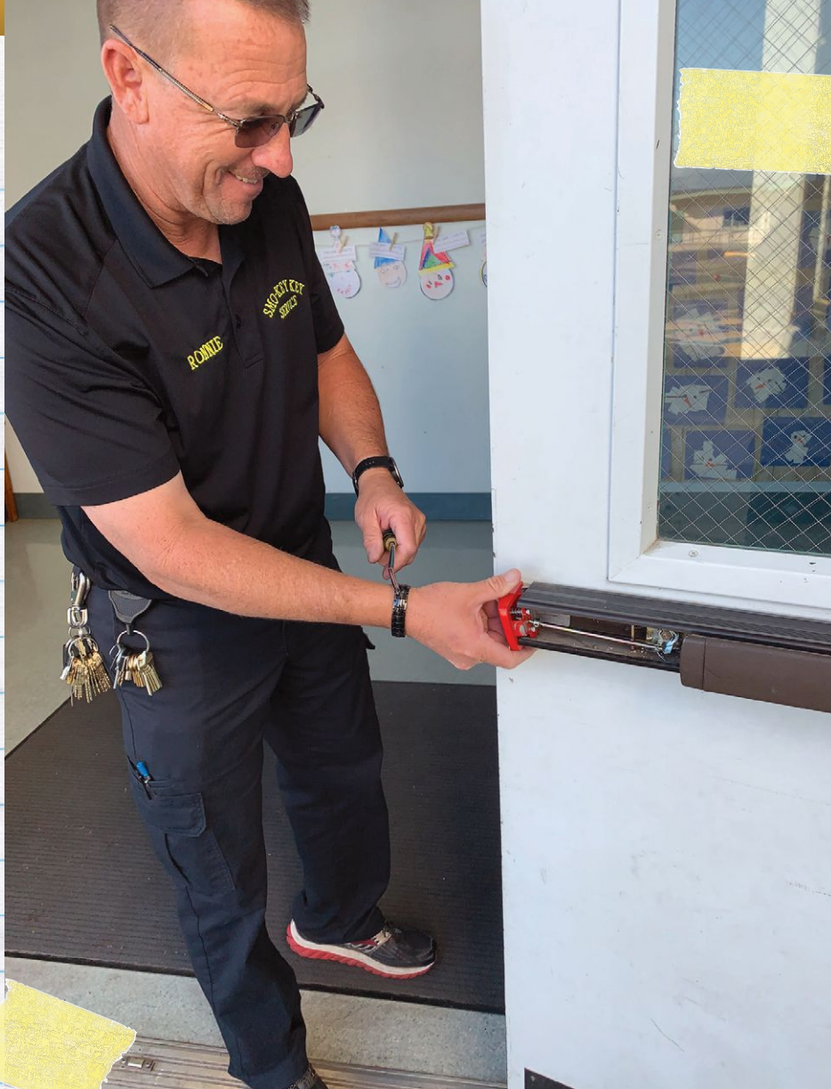
Ronnie Rehn with Smo-Key Key Service installs a red button lockdown device incorporated into the endcap of a panic device that is easy to find and engage.
