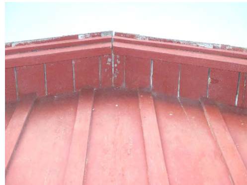
Figure 237: View of board-and-batten siding and tongue-and-groove boards that remain intact below the both sides of the building's roof. Photograph taken 6/25/2019.
