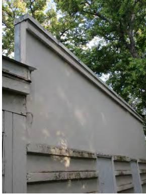
Figure 76: Western elevation of ROP Classroom (Utility Building/Garage), showing original parapet, coping, fascia, and three embossed horizontal bands. Photograph taken 6/24/2019.
