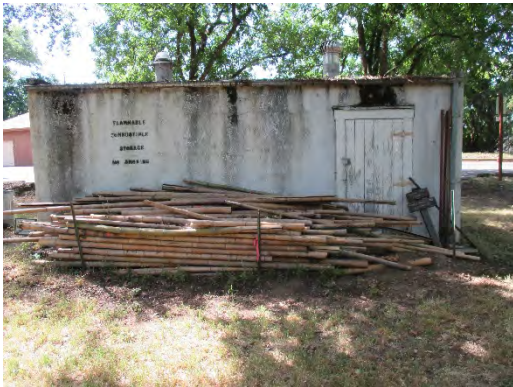
Figure 115: Northern elevation of Saw/Paint Storage Building (Fumigation Storage), with materials storage in foreground. Photograph taken 6/25/2019.
