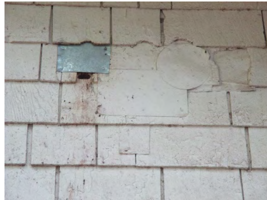
Figure 63: Detail of eastern elevation siding where once may have been an exit for a stovepipe exhaust. Photograph taken 6/24/2019.
