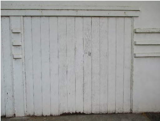
Figure 86: Enclosed vehicle bay door on southern elevation of ROP Classroom (Utility Building/Garage). Note wooden drop-siding used and its similarity to drop-siding on exterior shed. Photograph taken 6/24/2019.
