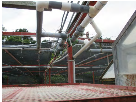
Figure 160: Close-up of valves for water-delivery system on interior of shadehouse. Photograph taken 6/25/2019.
