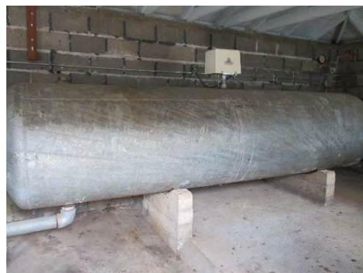
Figure 105: Large water tank located in interior of Tankhouse (Pumphouse). Photograph taken 6/25/2019.
