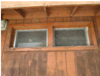
Figure 163: single-paned paired window sets with metal casings and wooden frames and mullions, located just below the eave on the northern elevation. Photograph taken 6/25/2019.
