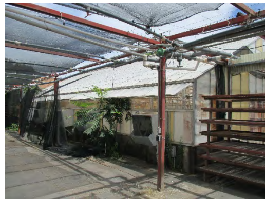
Figure 143: Western elevation of greenhouse, fitted with large jet-fan appliances. Shadehouse in foreground. Photograph taken 6/25/2019.
