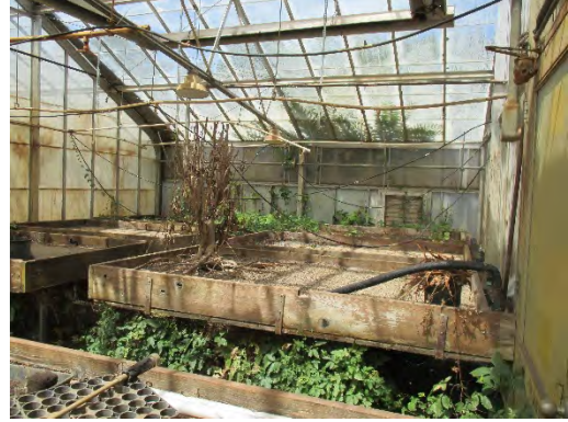
Figure 145: Another view of smaller north room of interior of greenhouse. Photograph taken 6/25/2019.
