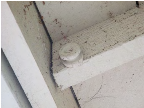
Figure 60: Pre-1940 ceramic insulator screwed into exposed rafter of Office Annex Building. Photograph taken 6/24/2019.
