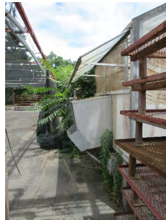
Figure 138: Window panes opened outwards above jet-fan units on western elevation. Photograph taken 6/25/2019.
