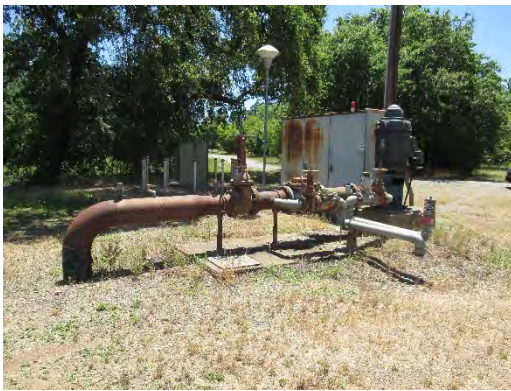
Figure 303: The north well, with storage cabinet and electric control box in the background. Photograph taken 6/26/2019.
