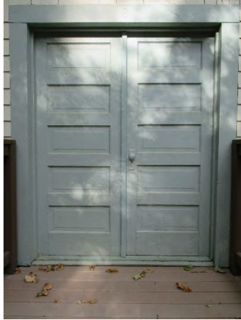
Figure 58: Front entrance to Office Annex Building, consisting of five-paneled wooden double-door. Photograph taken 6/24/2019.
