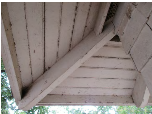
Figure 31: Older tongue-and-groove roof sheathing and rounded rafters under eave projection. Photograph taken 6/24/2019.
