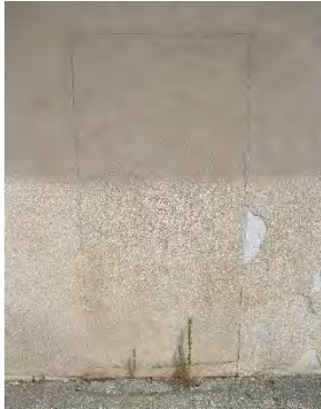
Figure 132: One of three blocked-in doorways on the southern elevation of headhouse. Photograph taken 6/25/2019.
