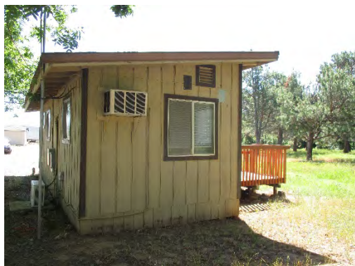
Figure 287: Western elevation with metal patches. Photograph taken 6/26/2019.
