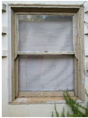
Figure 78: The only remaining functional window on the eastern elevation of the ROP Classroom (Utility Building/Garage). Note curvilinear motif at bottom of upper sash. Photograph taken 6/24/2019.
