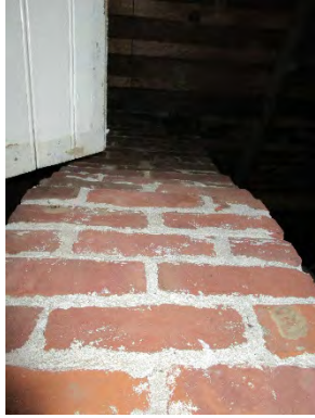
Figure 50: Original brick chimney, now truncated and no longer functional, but still accessible via an access chute in the ceiling of the present-day restroom. Photograph taken 6/24/2019.
