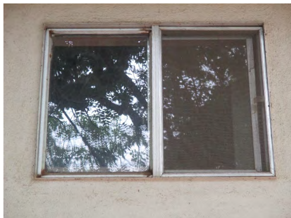
Figure 43: 1960s-era aluminum-framed horizontally sliding window. The only of this post-1950 type on the building. Photograph taken 6/24/2019.
