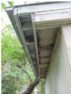
Figure 74: View of two roof construction periods atop exterior shed, built sometime after 1979, on northern side of ROP Classroom (Utility Building/Garage). Photograph taken 6/24/2019.
