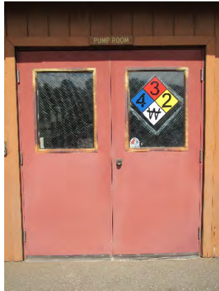
Figure 161: Double-door entrance to pump room on western elevation of Pump/Injector Building. Photograph taken 6/25/2019.
