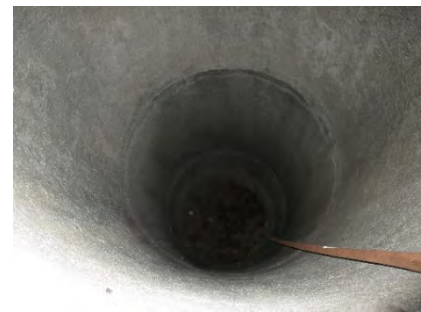
Figure 244: View looking into concrete irrigation standpipe south of Comanche Road, with manual operating mechanism descending into its depth. Photograph taken 6/25/2019.
