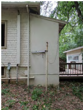
Figure 42: Northeastern corner of the building, showing eastern elevation of stucco-clad restroom/hallway addition. Photograph taken 6/24/2019.
