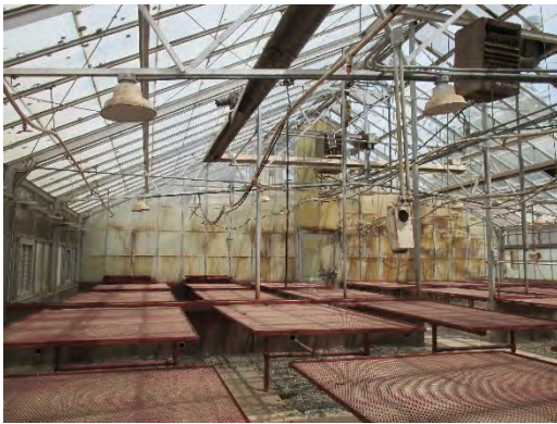
Figure 146: Larger south room of interior of greenhouse. Note concrete walkways interspersed with gravel to allow for water drainage within the building. Photograph taken 6/25/2019.
