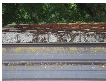
Figure 261: Detail of roofing materials of Shop Road small storage shed, with moss-covered asbestos shingles on upper pitch and corrugated sheet metal on lower pitch. Photograph taken 6/25/2019.
