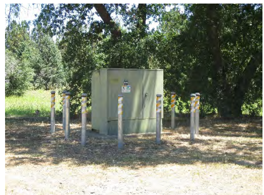
Figure 306: Adjacent electric control box on a concrete pad. Photograph taken 6/26/2019.
