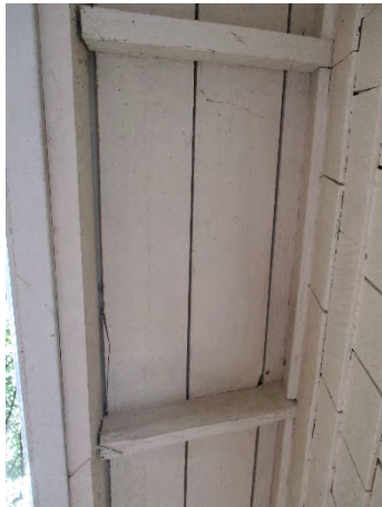
Figure 56: Original tongue-and-groove boards atop exposed rafters under the eave projection of the southern side of the Office Annex Building. Photograph taken 6/24/2019.
