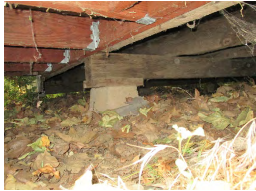
Figure 69: Underside of Office Annex Building, showing wooden beams atop a wooden shim atop a concrete pier foundation. Photograph taken 6/24/2019.
