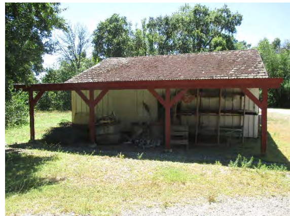
Figure 227: A thick mat of vegetative duff sits atop the northern portion of the Barn's roof. Photograph taken 6/26/2019.
