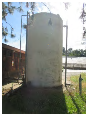
Figure 171: 10,000-gallon water tank. Photograph taken 6/25/2019.
