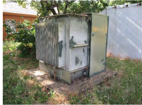
Figure 186: Back-side of large electric control box. Tree Cooler 2 of 3 in background. Photograph taken 6/25/2019.
