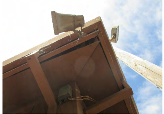
Figure 133: Under-eave projection, boxed in with plywood, showing utility pole and light fixtures at northeast corner of building. Photograph taken 6/25/2019.
