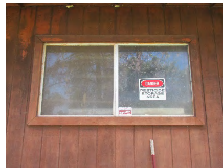
Figure 164: double-paned vertically sliding windows with metal casings and wooden frames, located about one foot below the eave of the eastern elevation. Photograph taken 6/25/2019.
