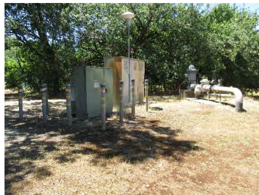
Figure 308: Electric control box and storage cabinet on left, south well on right. Photograph taken 6/26/2019.
