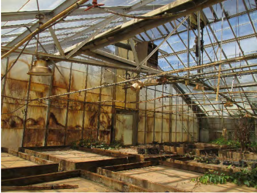
Figure 144: Smaller north room of interior of greenhouse, considerably deteriorated with uncontrolled vegetative growth. Photograph taken 6/25/2019.
