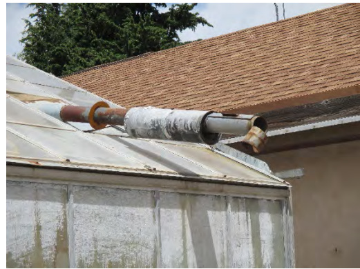
Figure 147: Disconnected water delivery system at northeast corner of greenhouse. Photograph taken 6/25/2019.
