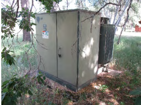
Figure 185: Front-side of large electric control box. Photograph taken 6/25/2019.
