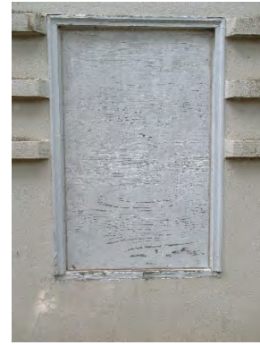
Figure 79: Boarded-up window on the western elevation of the ROP Classroom (Utility Building/Garage). Photograph taken 6/24/2019.
