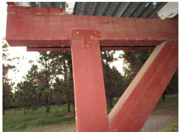
Figure 231: Metal T-brace attaching wooden beams of porch addition. Photograph taken 6/25/2019.
