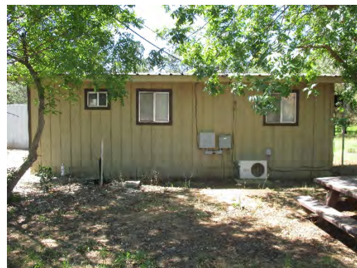
Figure 286: Northern (roadside) elevation with utility connections. Photograph taken 6/26/2019.
