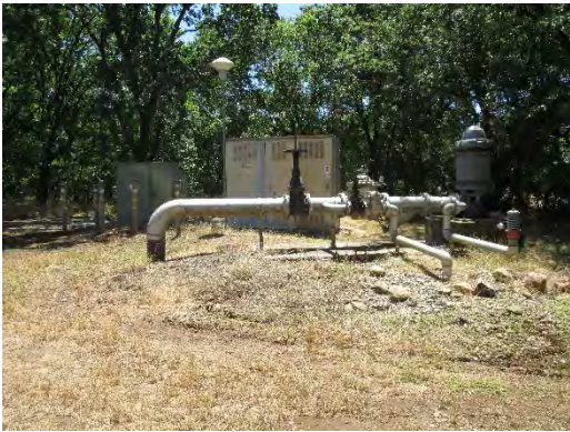
Figure 307: The south well, with storage cabinet and electric control box in the background. Photograph taken 6/26/2019.
