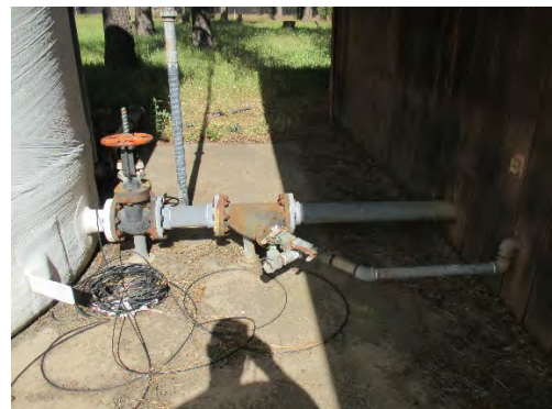
Figure 172: Water-delivery connections from water tank into Pump/Injector Building. Photograph taken 6/25/2019.
