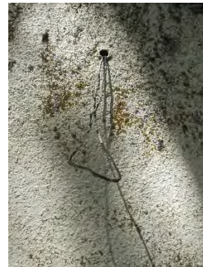
Figure 118: Remains of exterior electrical wiring that once serviced an exterior light on the eastern elevation of the building. Photograph taken 6/25/2019.
