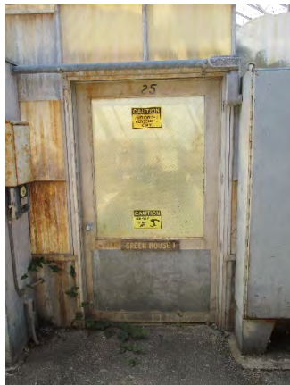
Figure 137: Main door, northern elevation across from the propagation area/potting room of the headhouse. Photograph taken 6/25/2019.
