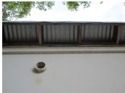
Figure 75: Southern eave projection of ROP Classroom (Utility Building/Garage), with tubular hole below. Photograph taken 6/25/2019.
