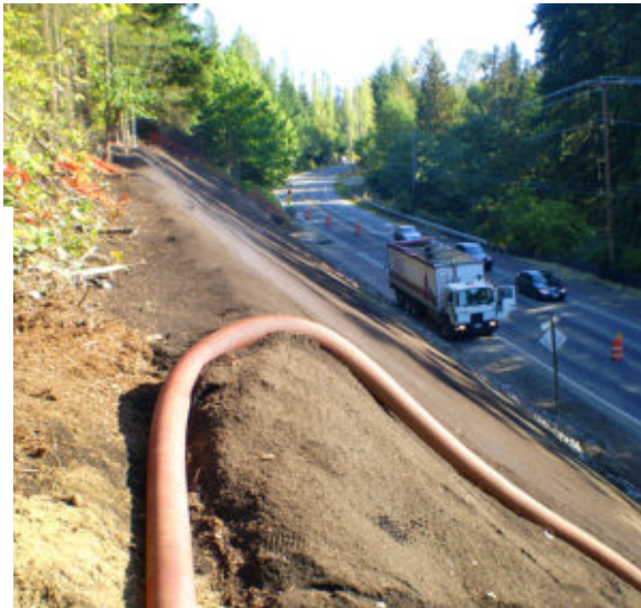
Opening photo (top of page): Slope with completed treatments and temporary irrigation system. (Above) Application of compost blanket Photos courtesy of Caltrans
