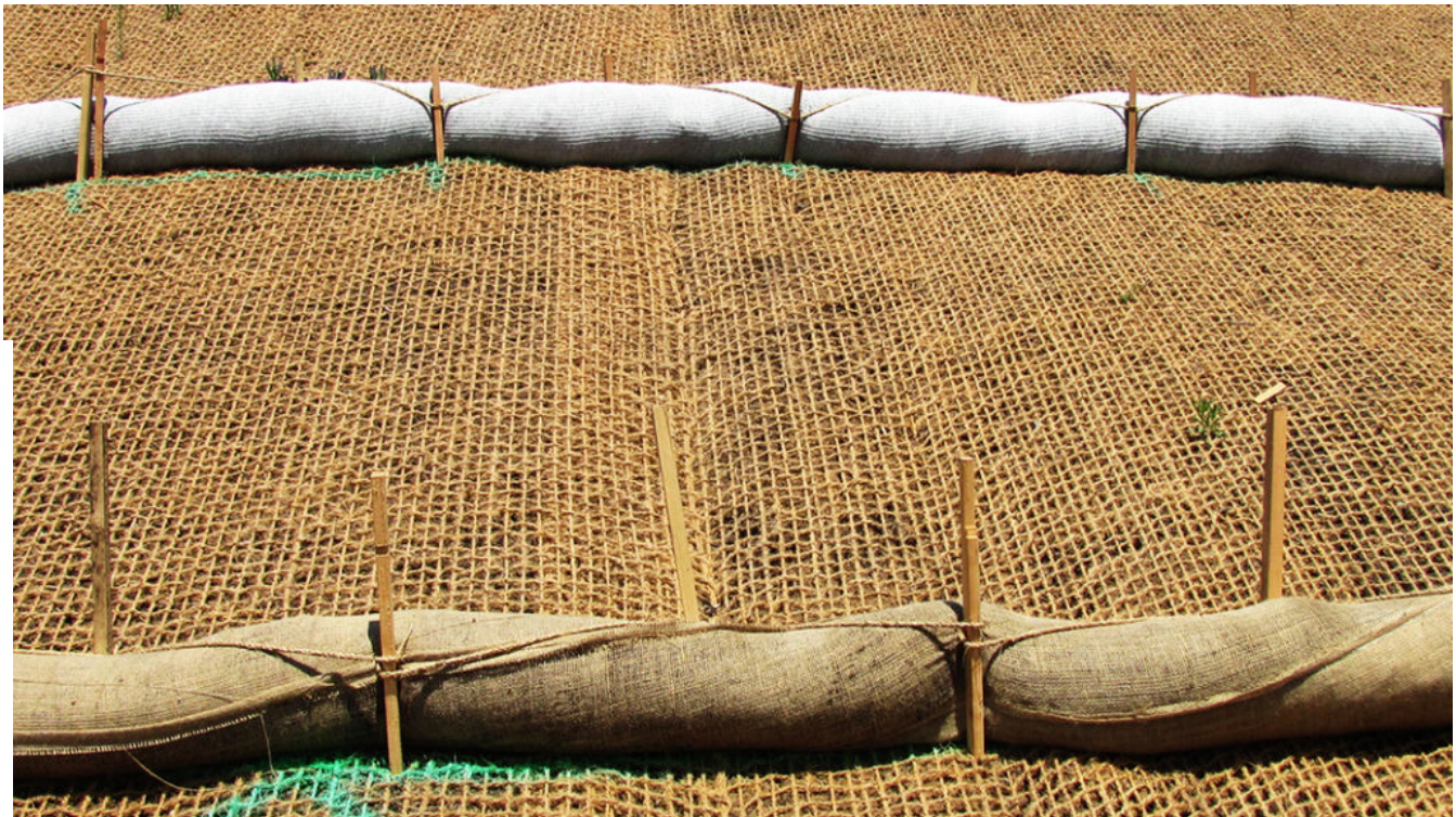
Utilization of compost socks on slope in California Photo courtesy of Caltrans
