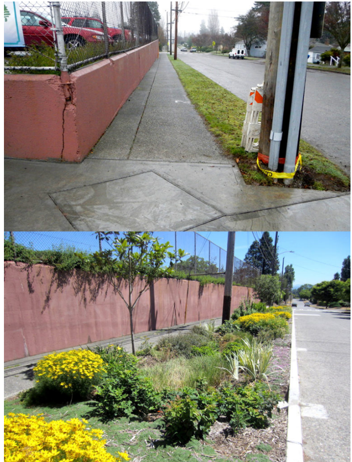
Biofiltration strip constructed in King County, Washington — before (top) and after (above).
