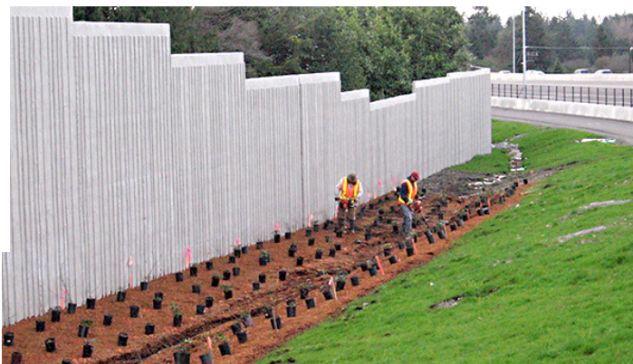
Construction of vegetative swale in Washington State (top photo and above). Photos courtesy of Craig Cogger, Washington State University
