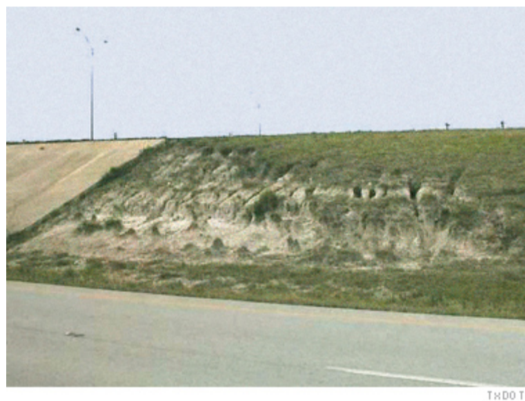
(Before) Erosion along State Highway 47 in College Station, TX, threatens this riprap slope. Left alone, the erosion would be expensive to repair.
