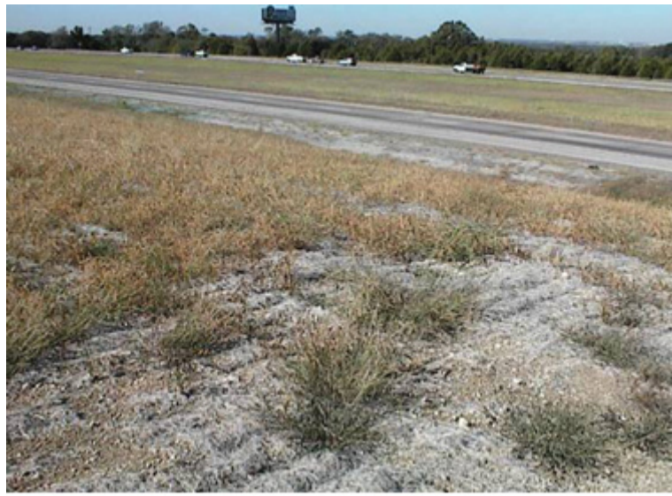
These soil erosion blankets along Spur 208 in the Dallas area failed to establish grass.
