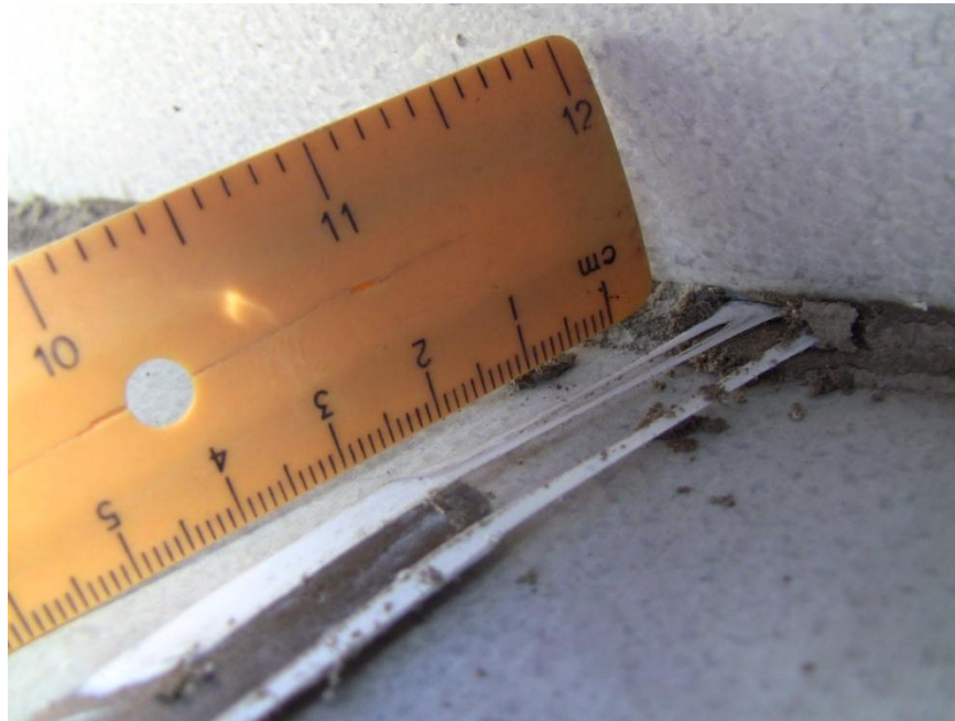
Figure 15 – Sealant between metal panel and metal ridge closure was also very elastic after 31 years in Wyoming.
