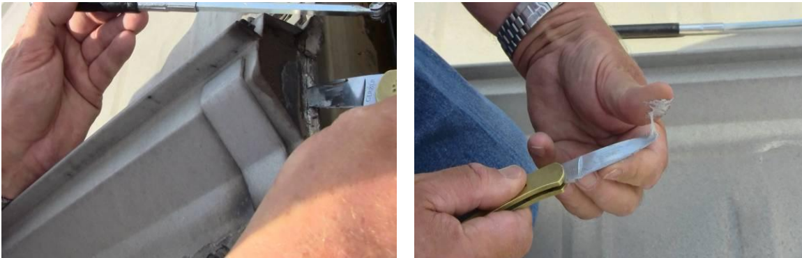
Figure 14 – Eave closure probed with knife edge (left) produced a sample of the butyl sealant that exhibited significant elasticity after 33 years in Denver (right).
