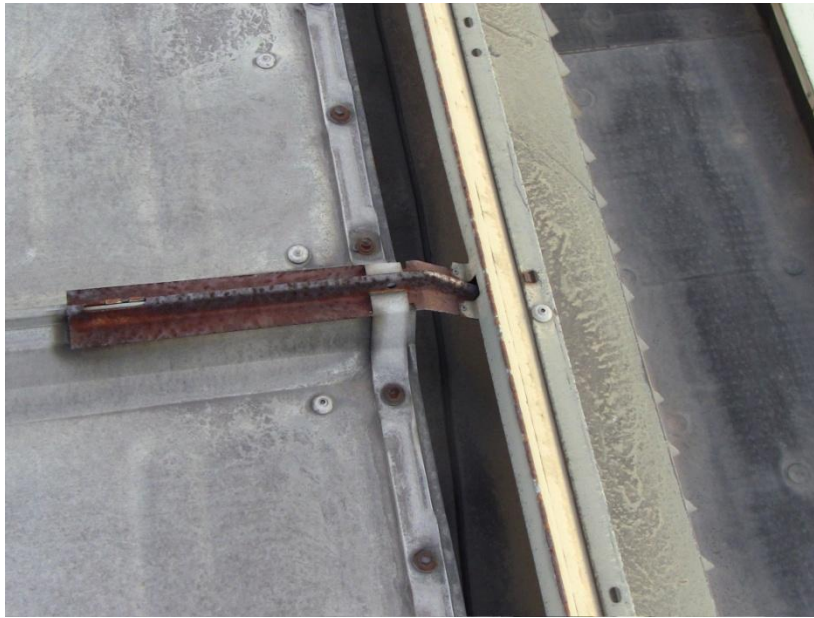
Figure 23 – Gutter hangar performance of galvanized G-90 steel after 32 years in Ohio.
