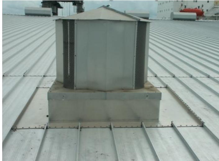
Figure 4 – Best-practice floating equipment curbs.
