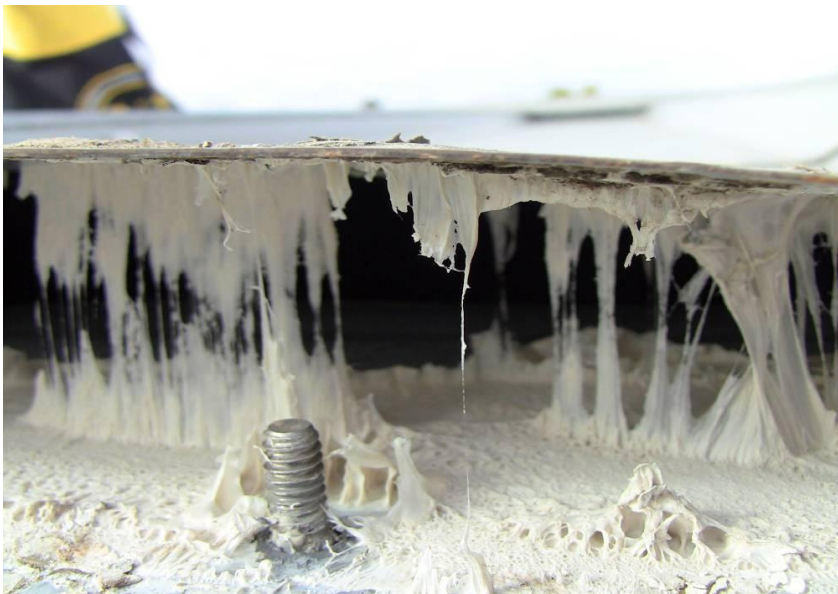
Figure 13 - Excellent elasticity demonstrated by the butyl sealant on the Denver roof after 33 years.
