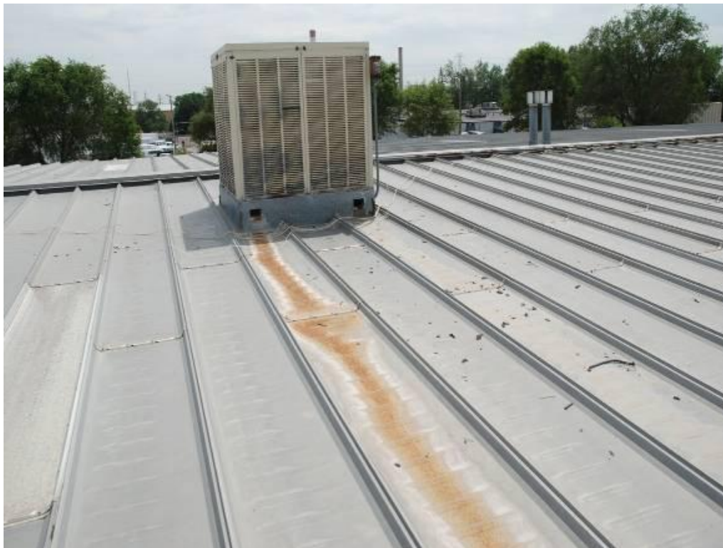
Figure 20 – Accelerated corrosion of 55% Al/Zn sheet due to improper drainage of copper ion-containing HVAC condensate.
