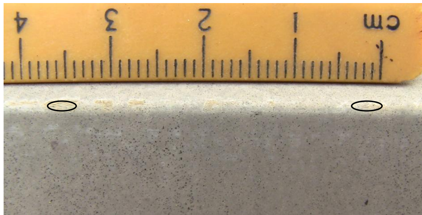
Figure 11 – Light crazing and superficial staining along a major rib profile radius after 29 years’ exposure on a roof in Athens, GA.
