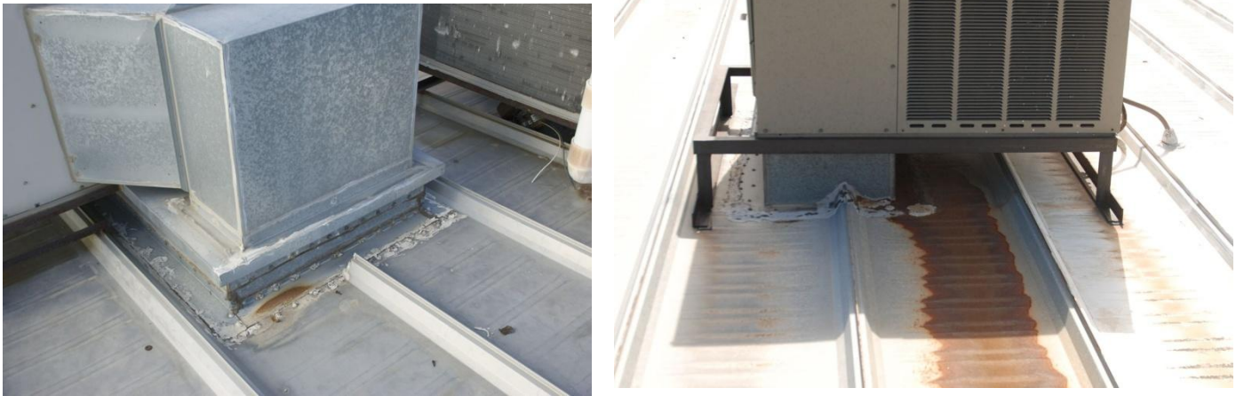
Figure 21 – Typical examples of poor HVAC mounting.
