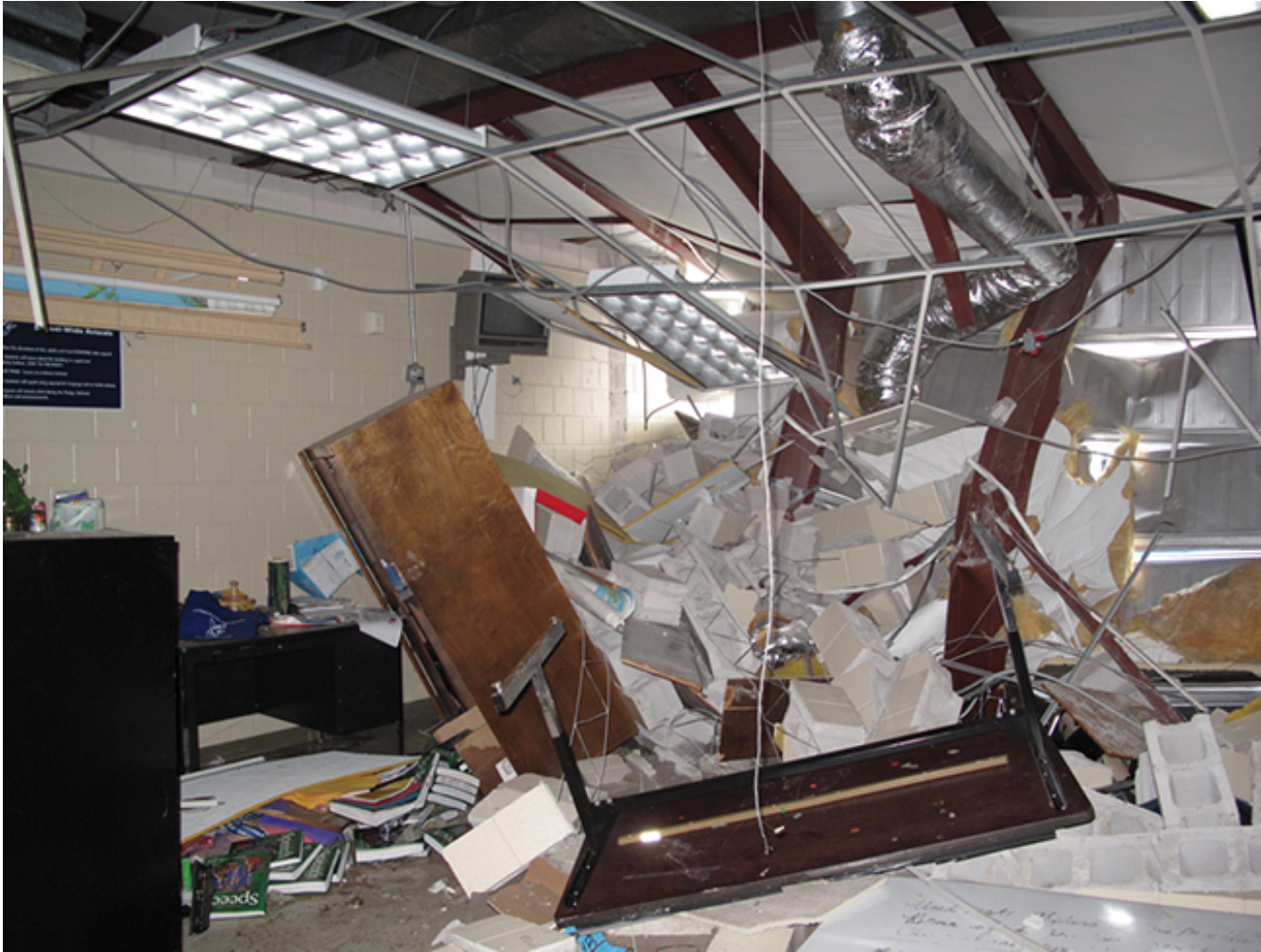
Figure 7: Re-cover roof structure failure—interior
