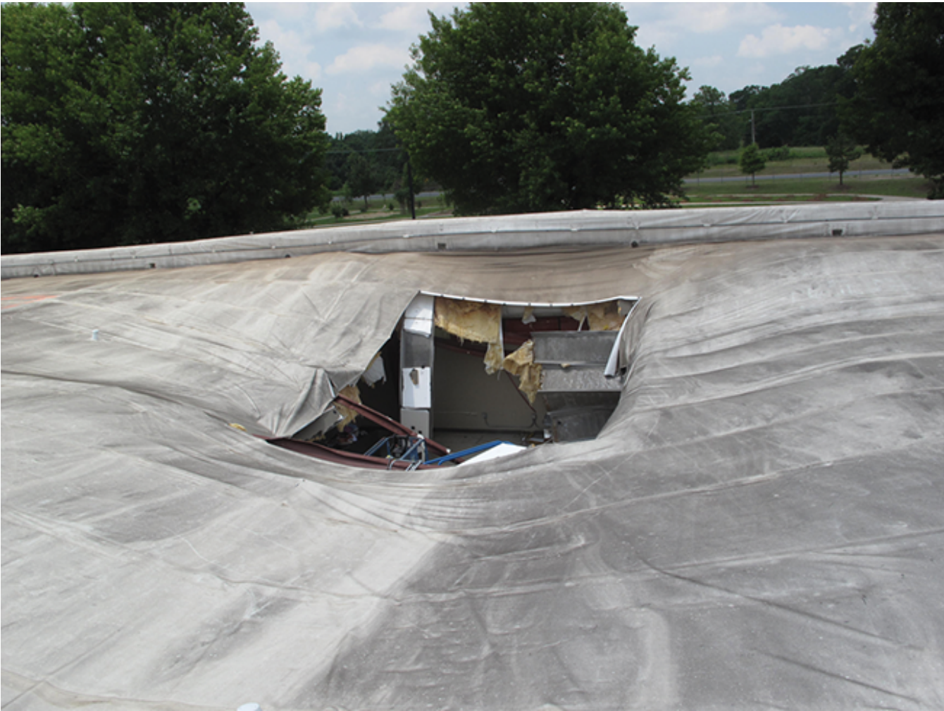
Figure 6: Re-cover roof structure failure—exterior
