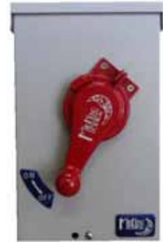
Figure 14 Combiner/ Breaker box with single power switch
