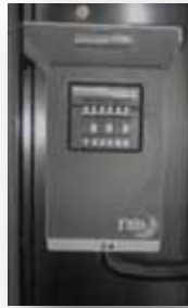
Figure 15 Combiner/ Breaker box, accessing breakers
