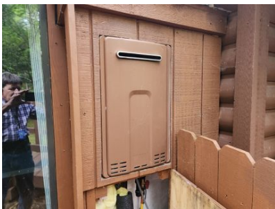
Exterior tankless water heater
