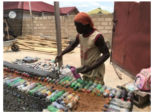
Spread the mortar on the wall and continue to lay the bricks.
