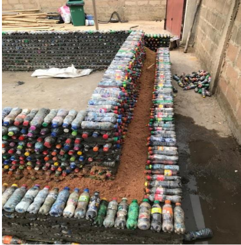
Fill in between the two walls with treated saw dust as shown.
