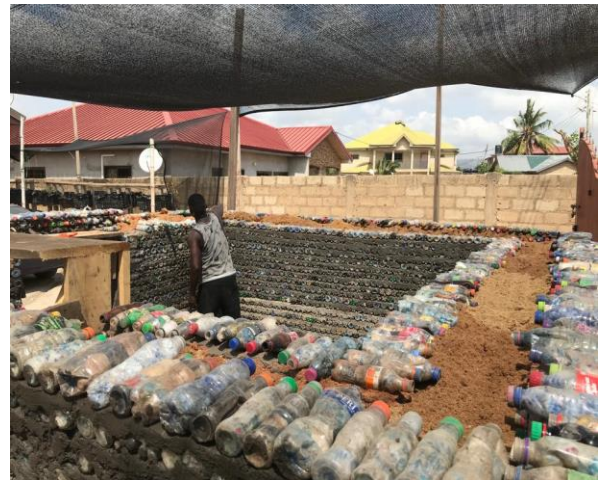
Pack in between the two walls with treated saw dust as shown
