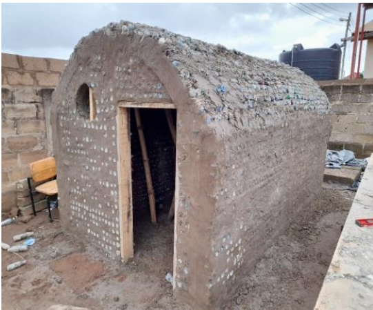
Carefully lay EcoBricks on top of the \frac{1}{2} " wire to form the roof as shown.
