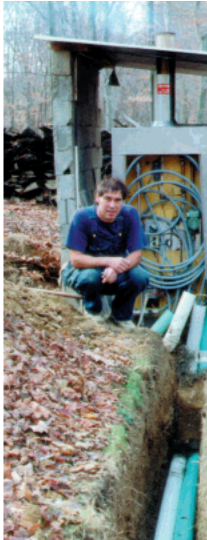
The stove sets on a concrete pad in a small shed. The trench connects it to the barn. The shed make it nicer when filling the stove in bad weather.
