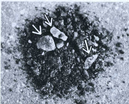
Figure 1-4. Arrows indicate deteriorated mortar that has come loose with the creosote during routine chimney cleaning. This is a sure sign of chimney problems.
