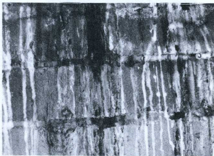
Figure 1-3. A close-up of a chimney with possibly terminal creosote damage. The acidic creosote has eaten away at the mortar joints, making them porous and a fire hazard.
