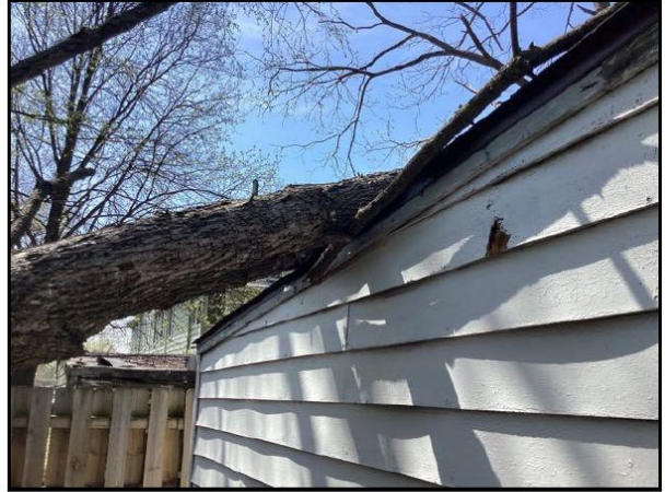
48. Trees or shrubs too close to building
