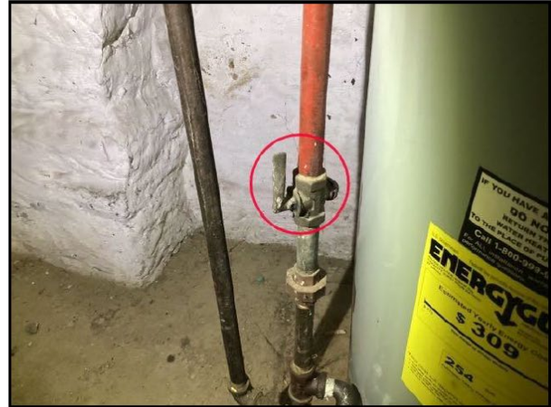
119. Older style gas shut off valves
