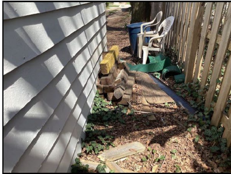
49. Wood pile too close to structure
