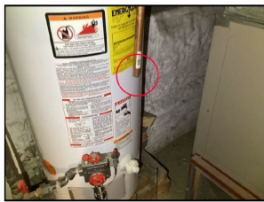
123. Discharge tube too short
