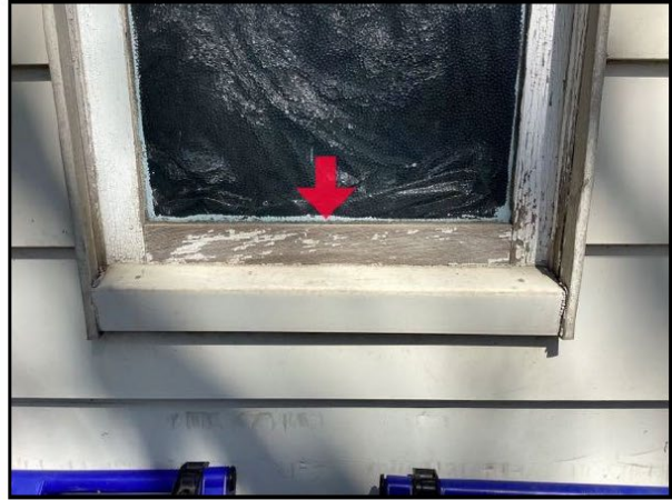
44. Paint or stain needed
