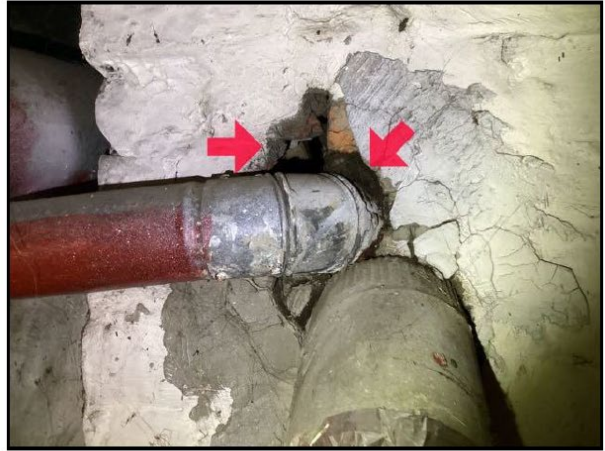
11. Not properly sealed at chimney
