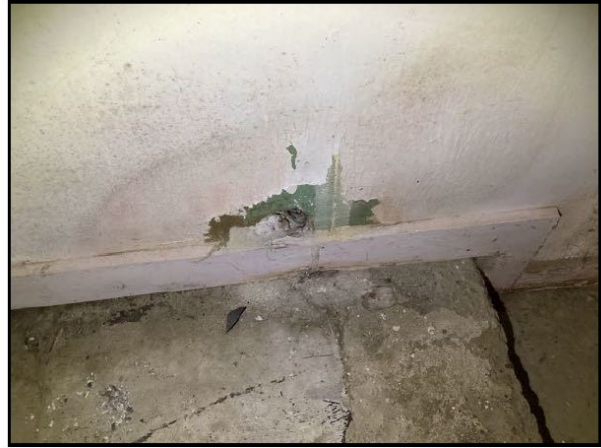
22. Crumbling plaster, dry wall or concrete walls
