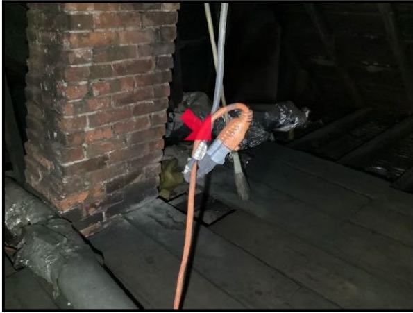
72. Extension cord used as permanent wiring
