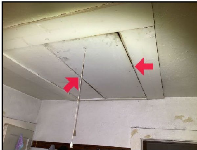
106. Not insulated / Weatherstripped
