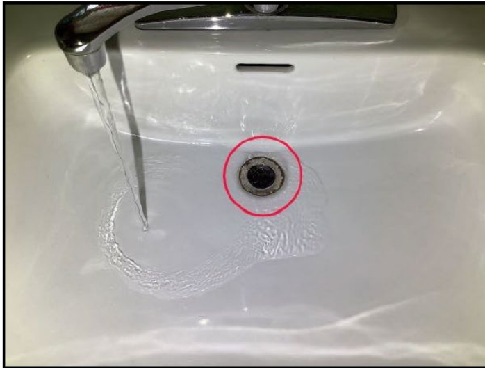
131. Drain stop missing
