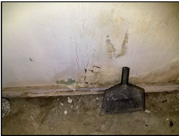
23. Crumbling plaster, dry wall or concrete walls
