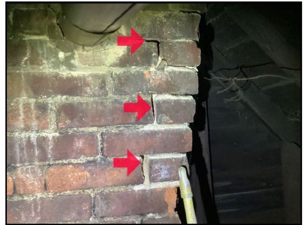
100. Loose, missing or deteriorated mortar
