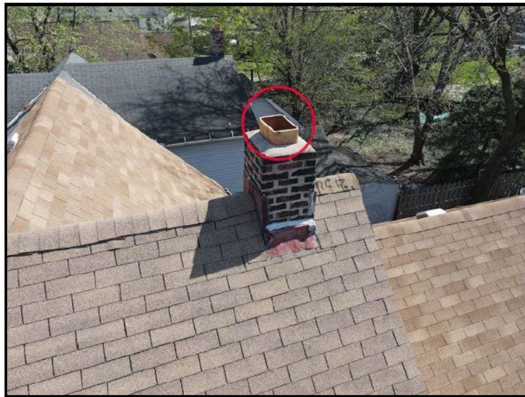
101. Rain cap missing or damaged
