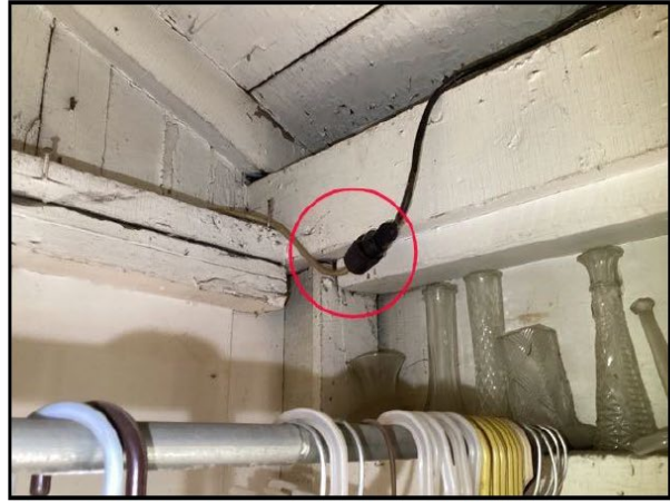
73. Extension cord used as permanent wiring
