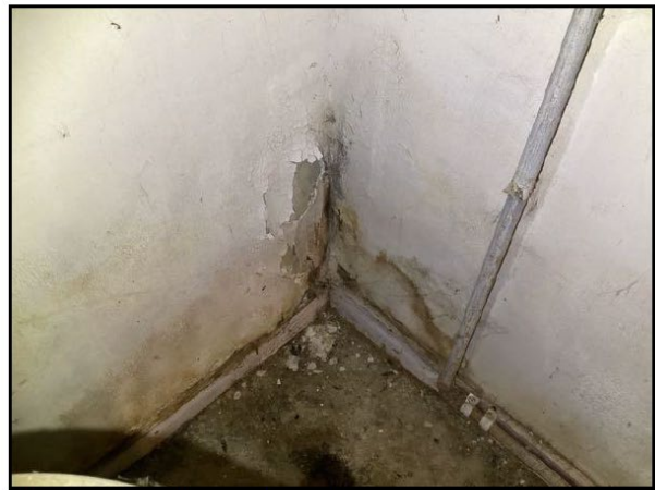
24. Crumbling plaster, dry wall or concrete walls
