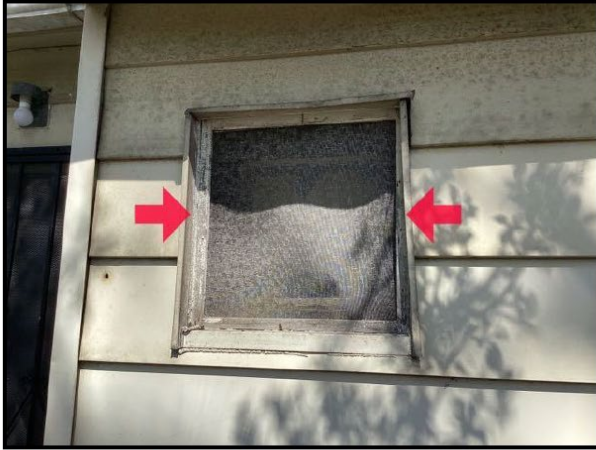
43. Paint or stain needed
