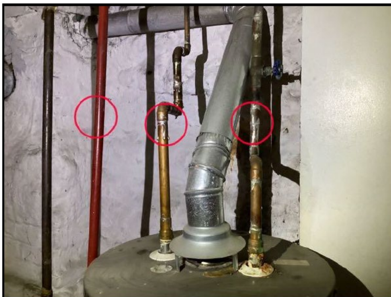
67. Missing bonding wire
