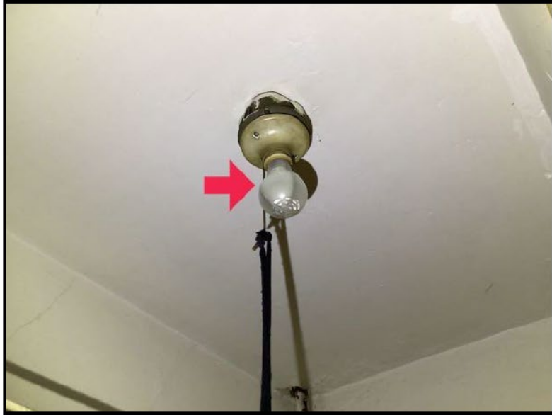
82. Improper closet lighting
