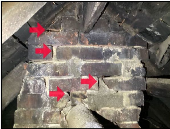
99. Loose, missing or deteriorated mortar
