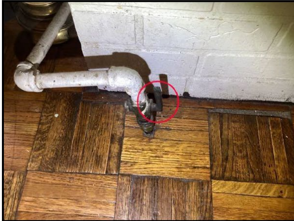
118. Older style gas shut off valves
