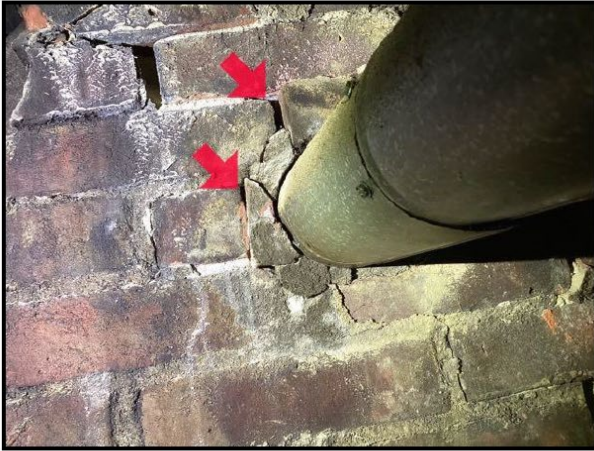
10. Not properly sealed at chimney
