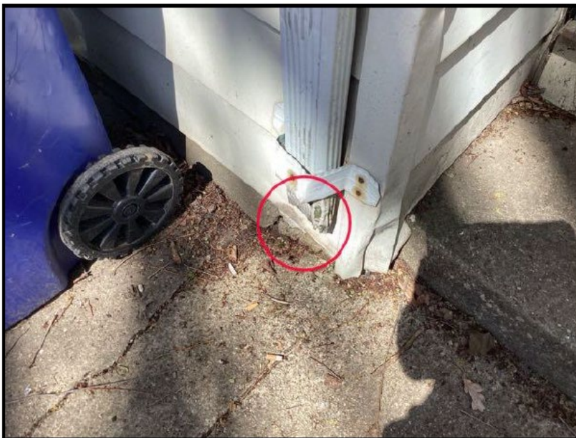
42. Discharge too close to building
