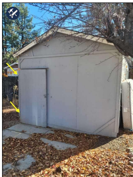
Hinges on the Door are placed in a strange place.
