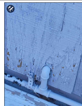
East Side--Peeling Paint Observed.
