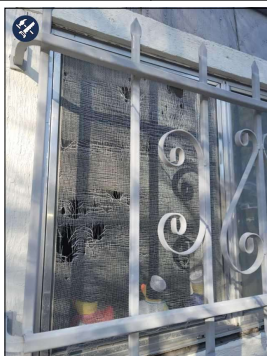
South Side--Screen Damaged
