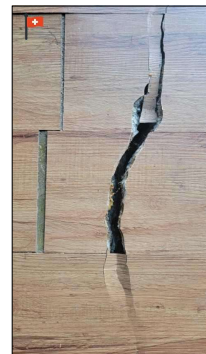
Living Room--Numerous Heavy Foundation Cracks Noted.
