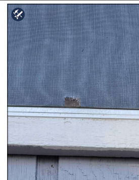
South Side--Upstairs hole in the Screen.
