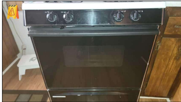
Could not Test, Gas Shutoff to Home at Time of Inspection.
