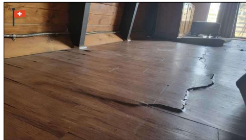
Dining Area--Numerous Heavy Foundation Cracks Noted.
