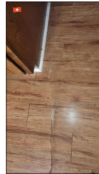
Numerous Heavy Foundation Cracks Noted.
