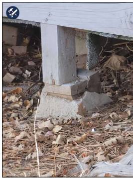
North Side--Instead of doing it right some just stacked block of Wood on top of the Failing footing to make do.
