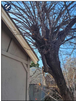
Tree is interfering with the Building.
