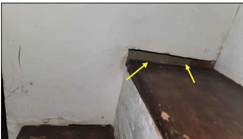
Holes Noted by Stairs.
