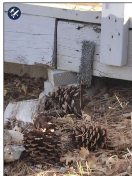
North Side--Fascia Board is twisting Supports are blocks of Wood
