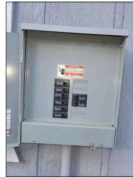
Sub-Panel on the South Side
