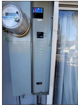
One 15 Amp in the Bottom of the Breakers
