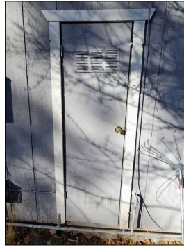
South Side Exterior Water Heater Closet
