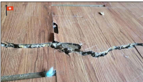
Living Room--Numerous Heavy Foundation Cracks Noted.
