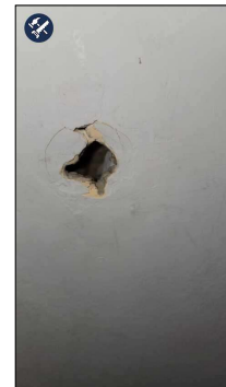
Entryway--Hole in Wall Caused by Doorknob.
