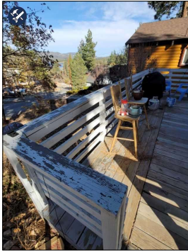
Railing is Loose
