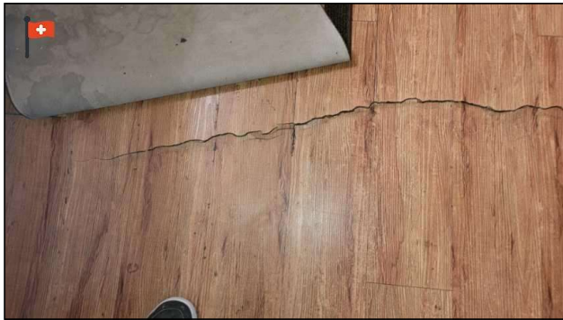
Numerous Heavy Foundation Cracks Noted.
