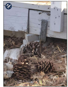
North Side--Fascia Board is twisting Supports are blocks of Wood
