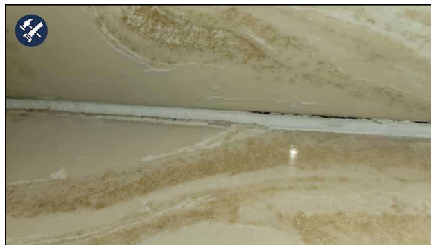
Upstairs Bathroom#2--Caulking Observed to be Cracking.
