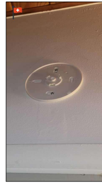
Bedroom#1--Smoke Detector Missing.
