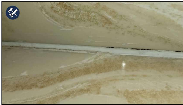
Upstairs Bathroom#2--Caulking Observed to be Cracking.
