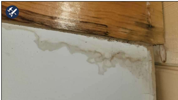
Bedroom#1, Inside Closet--There is evidence of moisture entering structure. We recommend contacting a contractor experienced in exterior systems to evaluate the area and suggest repair options.
