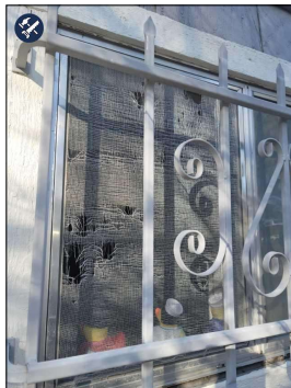
South Side--Screen Damaged
