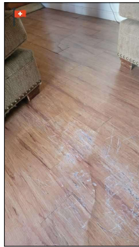
Living Room--Numerous Heavy Foundation Cracks Noted.
