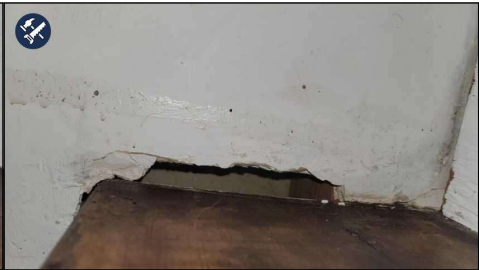
Holes Noted by Stairs.
