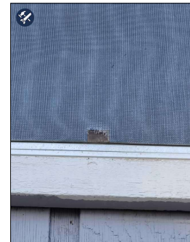
South Side--Upstairs hole in the Screen.
