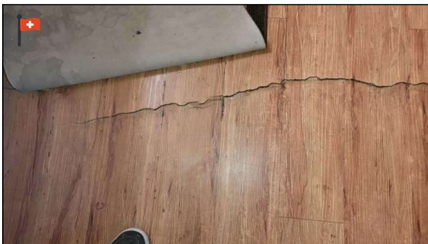
Numerous Heavy Foundation Cracks Noted.
