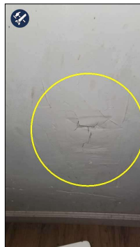
Past Repair Noted.
