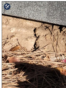
West Side--Crack in the Perimeter Wall
