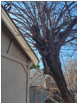
Tree is interfering with the Building.
