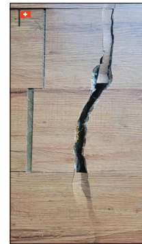
Living Room--Numerous Heavy Foundation Cracks Noted.
