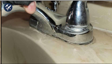
Bathroom#1--Faucet Observed Loose.
