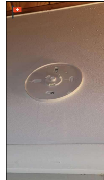
Bedroom#1--Smoke Detector Missing.
