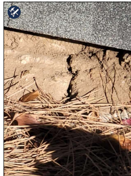
West Side--Crack in the Perimeter Wall
