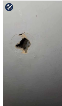
Entryway--Hole in Wall Caused by Doorknob.
