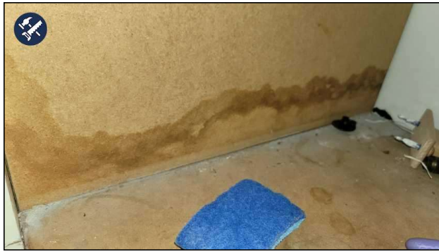
Upstairs Bathroom#2--There appears to be water damage under sink. This tested dry at the time of the inspection, but monitor for any further intrusion.
