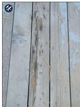
North Side Deck--Floor Boards are Showing Peeling Paint & Bare Wood Observed.
