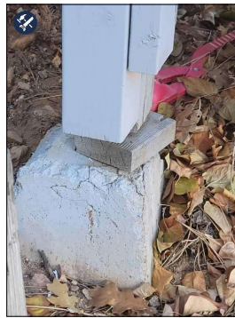
Northeast Corner--Barely sitting on the wood that was put on top of the Falling Apart Footing
