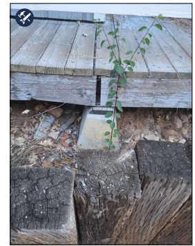
East Side--The Deck is Sagging at this point. May have to do with the Footing that are Cracked, crumbling, tilted and so on.
