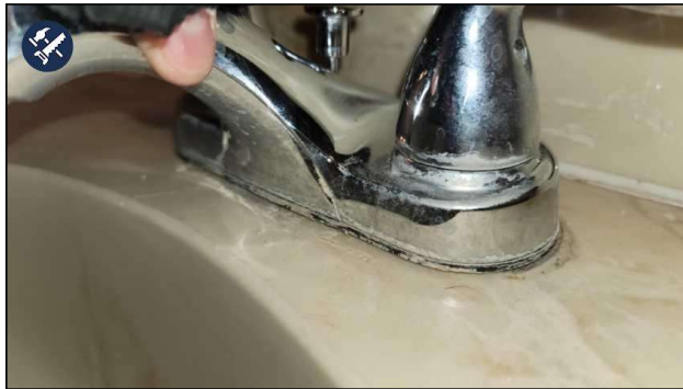
Bathroom#1--Faucet Observed Loose.
