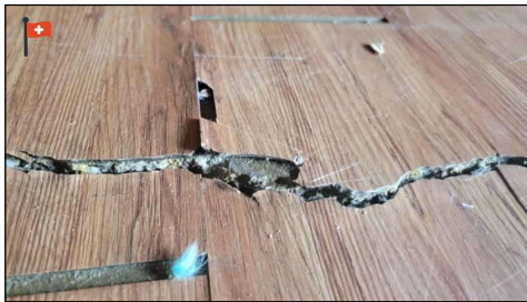
Living Room--Numerous Heavy Foundation Cracks Noted.
