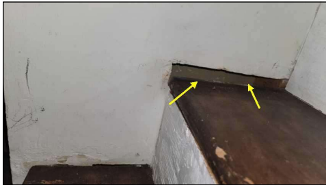
Holes Noted by Stairs.
