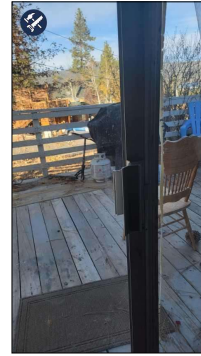
Living Room--Door is difficult to operate, this presents a safety hazard in the event of an emergency/fire. Recommend repair/adjusting of door by a Qualified Contractor to allow easy and smooth operation.
