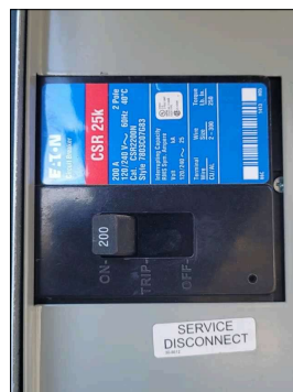
200 Amp Main Breaker
