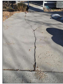
Crack in the Concrete
