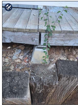
East Side--The Deck is Sagging at this point. May have to do with the Footing that are Cracked, crumbling, tilted and so on.
