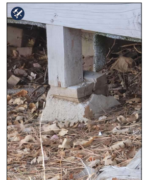
North Side--Instead of doing it right some just stacked block of Wood on top of the Failing footing to make do.
