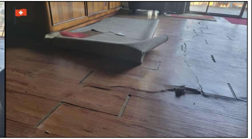
Living Room--Numerous Heavy Foundation Cracks Noted.
