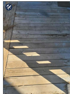
North Side Deck floor Boards are almost bare of wood.
