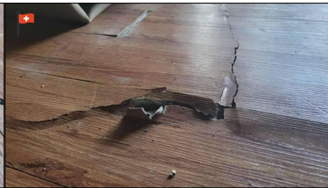
Living Room--Numerous Heavy Foundation Cracks Noted.
