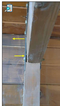
Living Room--Support Beam Observed to be Twisting.
