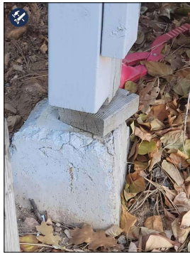
Northeast Corner--Barely siting on the wood that was put on top of the Falling Apart Footing
