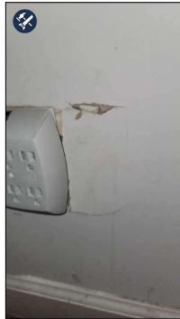
Dining Area--Damage to the Wall Observed(Cosmetic)
