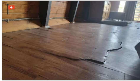
Dining Area--Numerous Heavy Foundation Cracks Noted.
