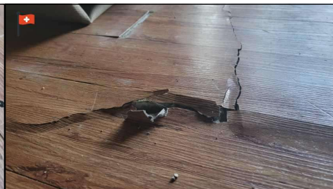
Living Room--Numerous Heavy Foundation Cracks Noted.
