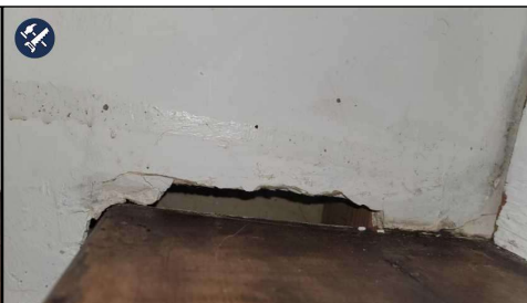
Holes Noted by Stairs.
