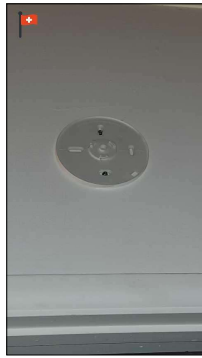
Bedroom#2--Smoke Detector Missing.
