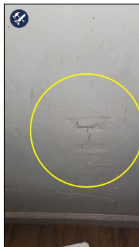
Past Repair Noted.
