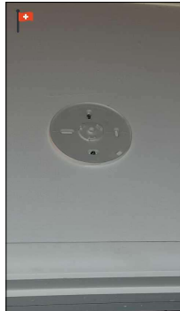
Bedroom#2--Smoke Detector Missing.
