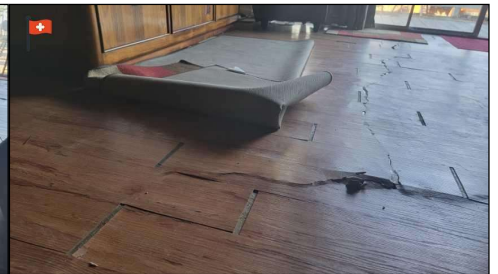
Living Room--Numerous Heavy Foundation Cracks Noted.
