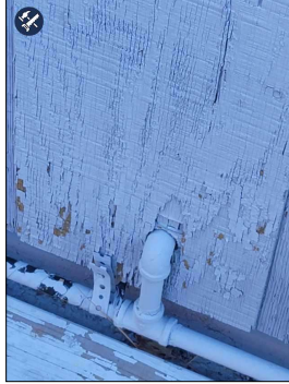
East Side--Peeling Paint Observed.
