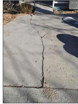
Crack in the Concrete
