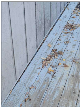
East Side--Gap is forming between the Deck & the Home. Recommend further evaluation by a Handyman for Answers & Options to this issue.
