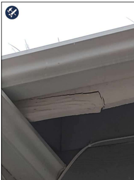
South Side--Crack in the Board
