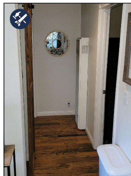
Hallway--In this Area there was a Smell in the hallway that actually smelled like a Dead rodent. Could not find and even when opened closet on the Left and the Crawlspace hatch was opened smell was not under there just in the Hallway.
