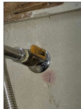
Water Supply Shut Off Valve for the Water Heater
