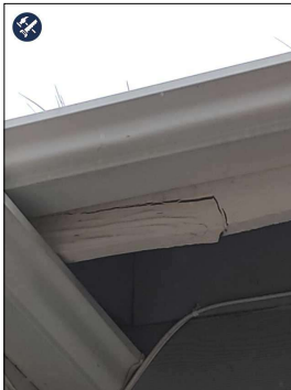
South Side--Crack in the Board
