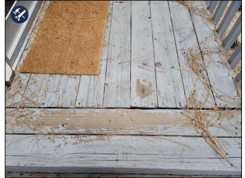
Deck Off of Bedroom#1--Floor Boards have Peeling Paint & Bare Wood Observed
