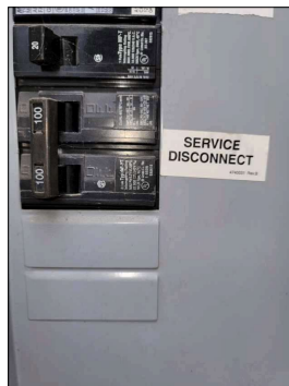
100 Amp Main Breaker
