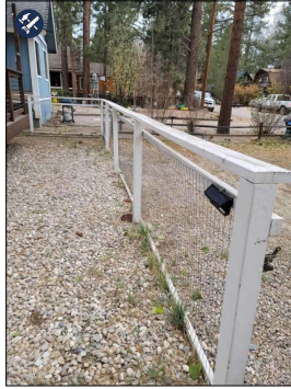
North Side is Shakey
