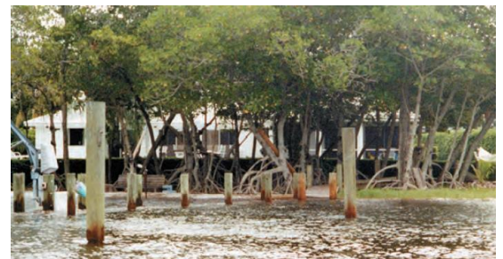
Undercutting with red mangrove
