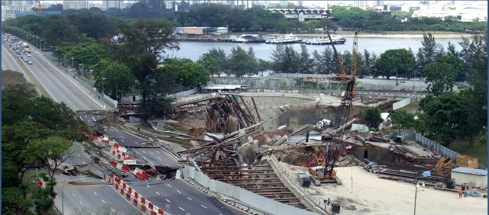
On April 20, 2004, a cave-in at the then Circle Line worksite caused a section of the Nicoll Highway to collapse.
