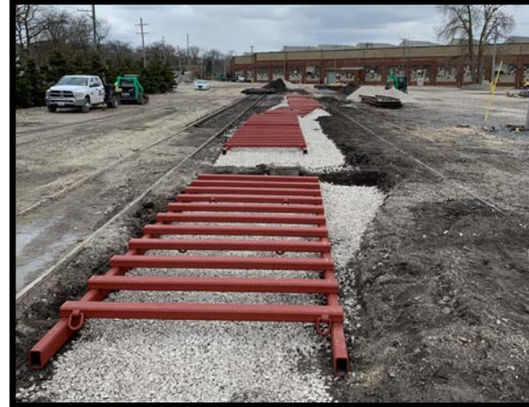
Set Ballast Frames, Match top of Rail elevations, dump rock in frames
