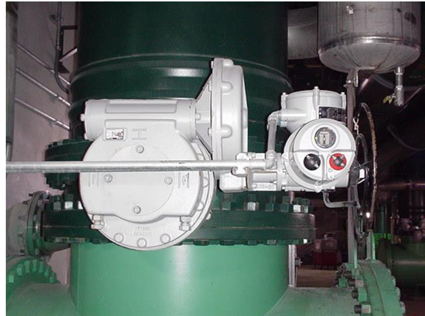
Filter Gallery Electric Actuator on Butterfly Valve
