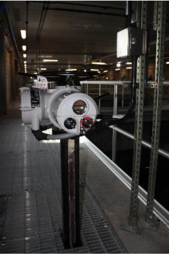
• Filter Influent Valve
