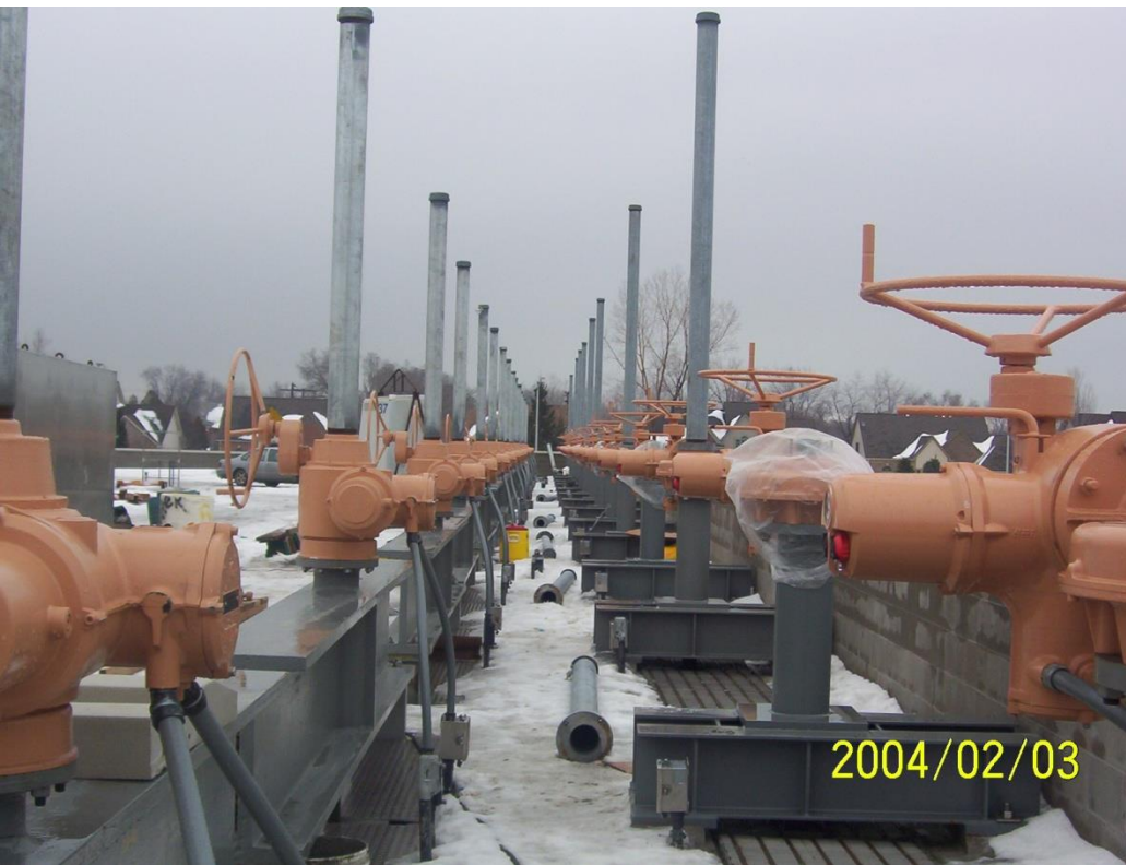
Electric Actuators On Gates
