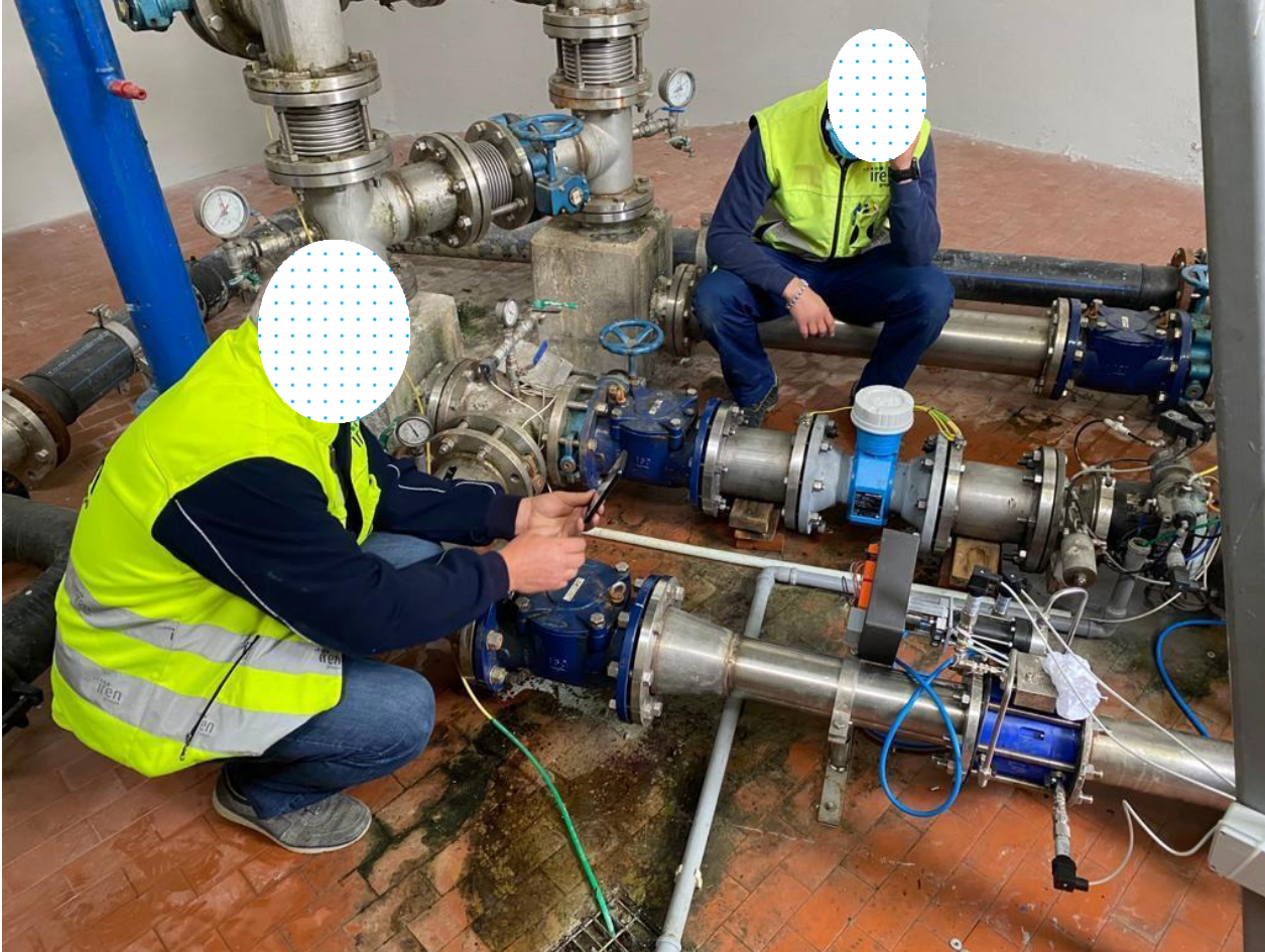
Installation with in-house controller
