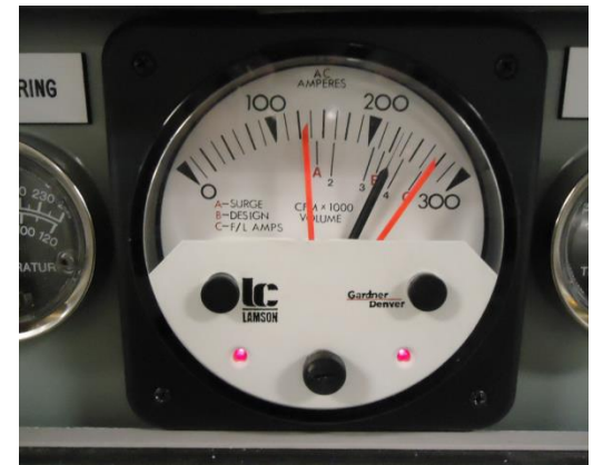
Ammeter readings above design
