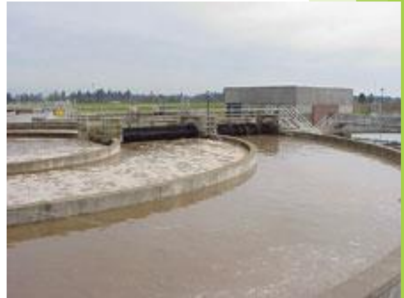
Wasting Aerobic the Bio-solids Removes Phosphorus
