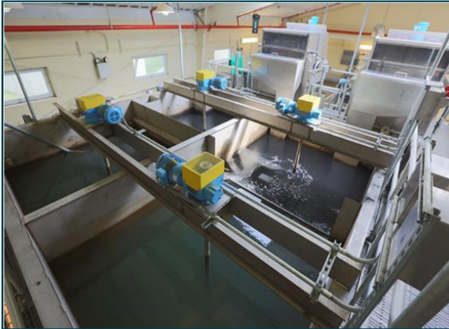
← Reaction Tanks and Magnetite Recovery Drums
