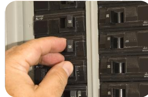
Manual and/or Building Automation
