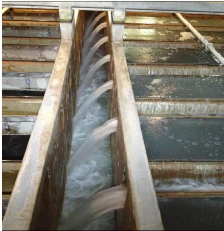
Filter under backwash
