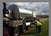
The delivery/insertion truck brings the ice slurry to the location and pumps the slurry into the forcemain.
