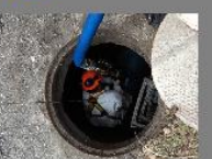
The slurry being pumped into the forcemain inside a casing at the cast-in-place.
