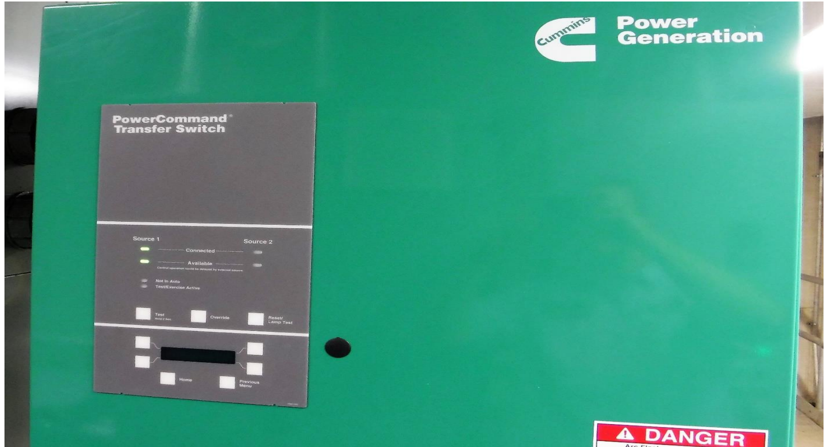
Transfer Switch at Dome
