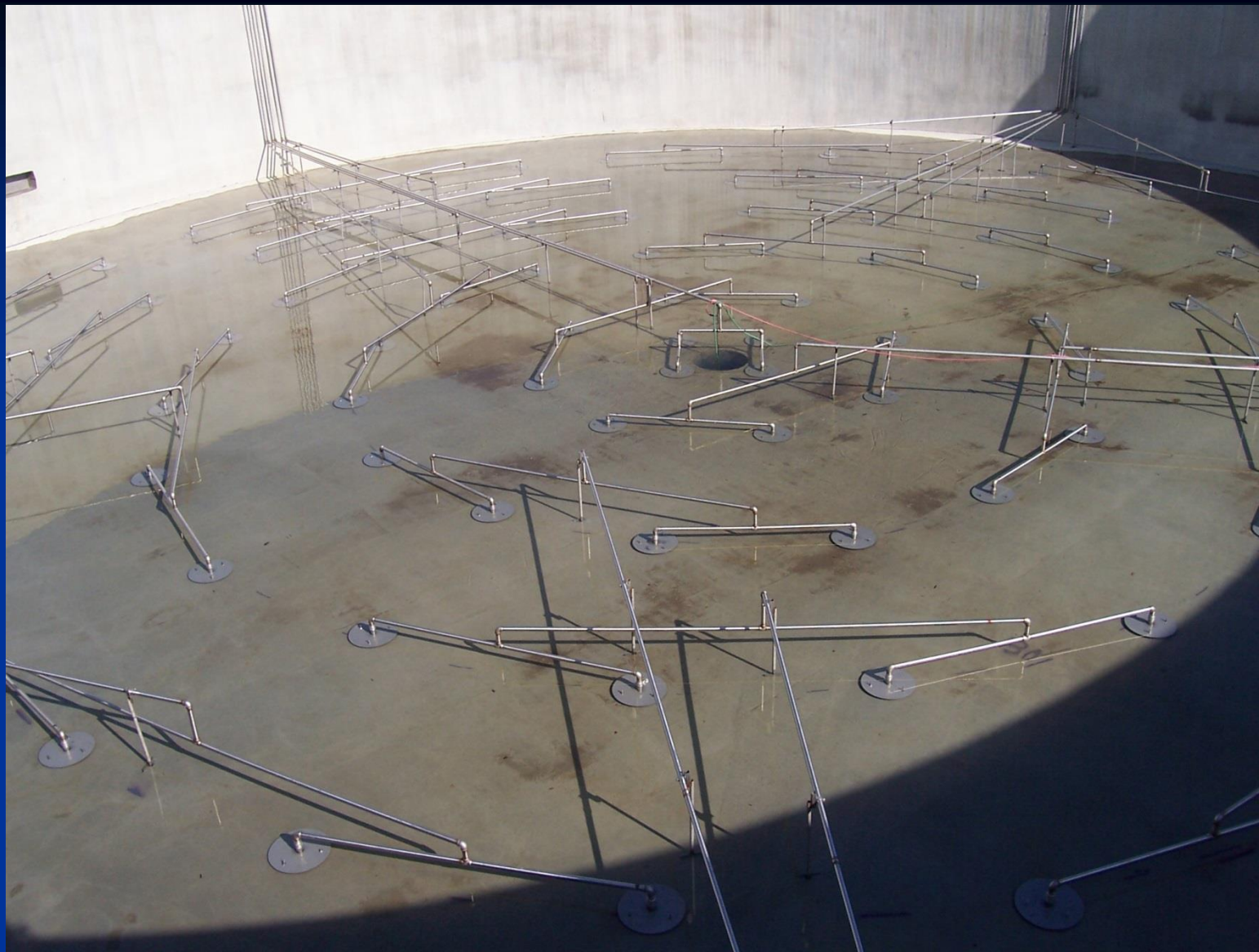
SS accumulator plates bolted to the floor of a 125ft diameter sludge tank
