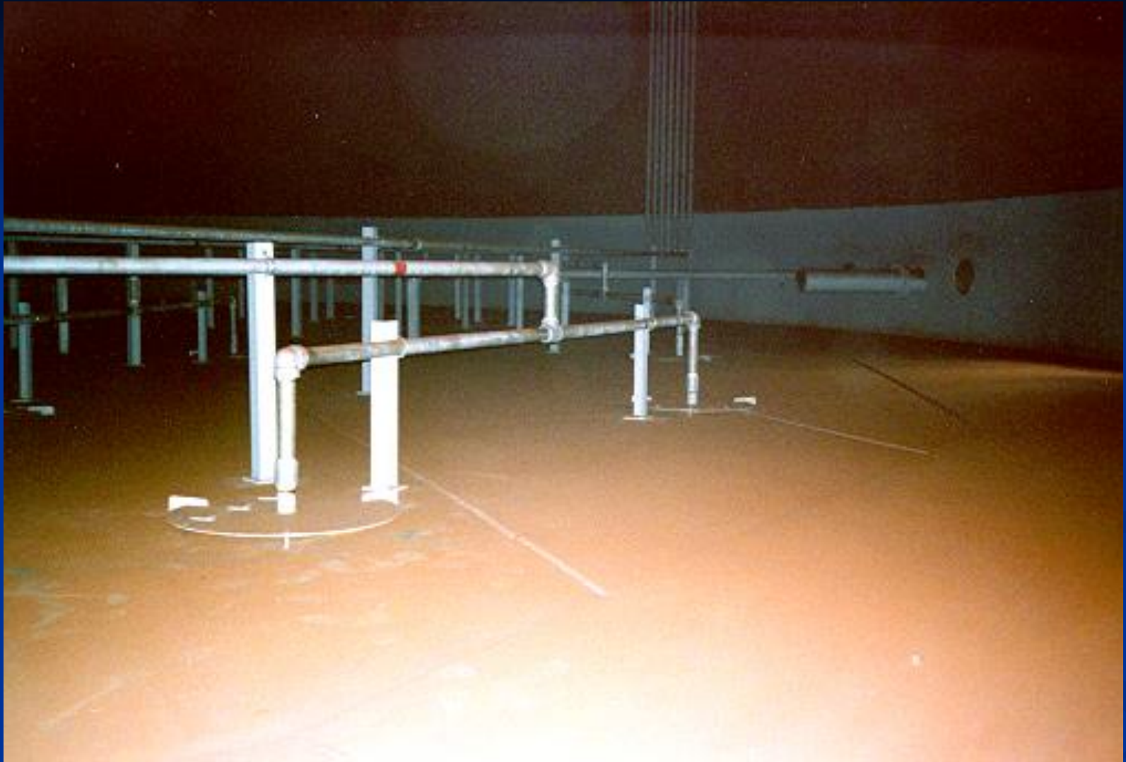
Accumulator plates on the floor of a 100ft diameter fuel storage tank
