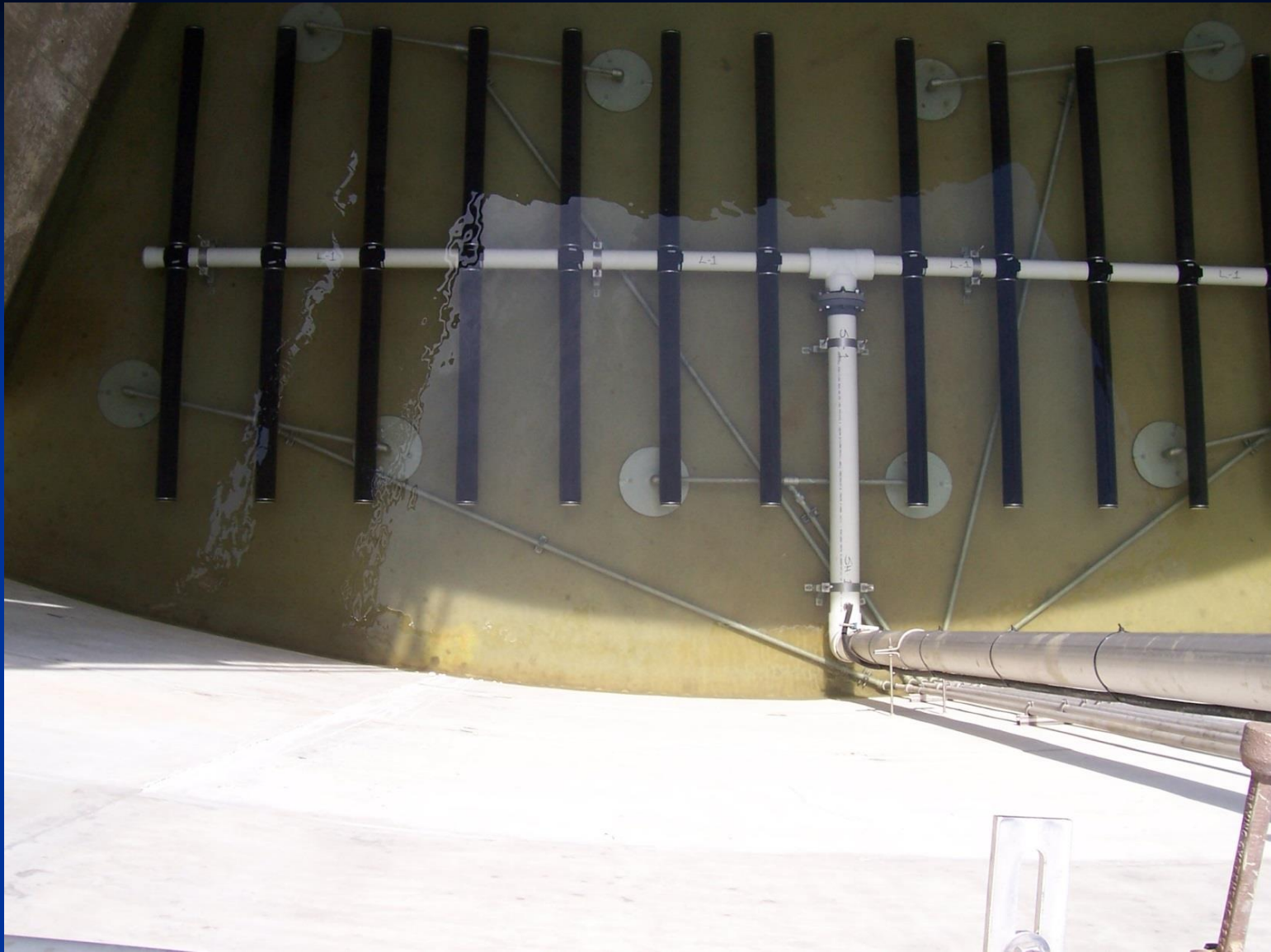
SS “double” plates bolted to the floor of an anoxic zone in an aeration basin
