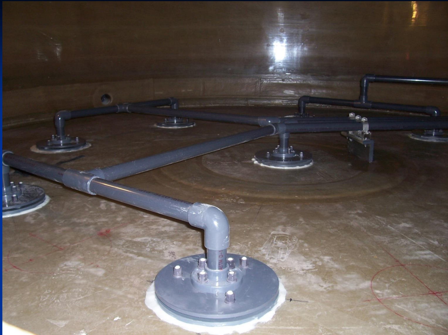
PVC “double” plates secured with epoxy to the floor of an FRP tank.
