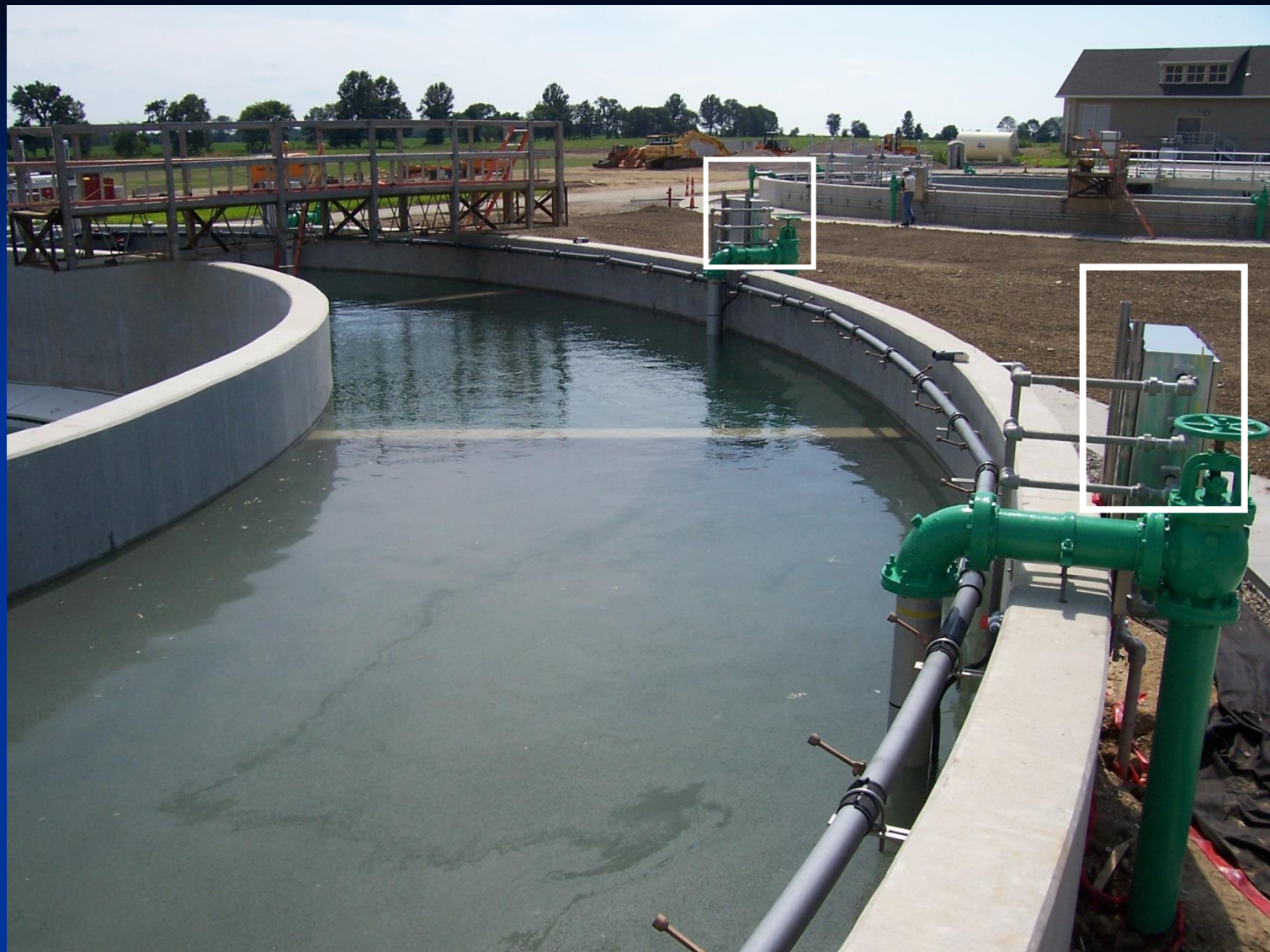
SS secondary enclosures mounted above anoxic zones at a municipal WWTP
