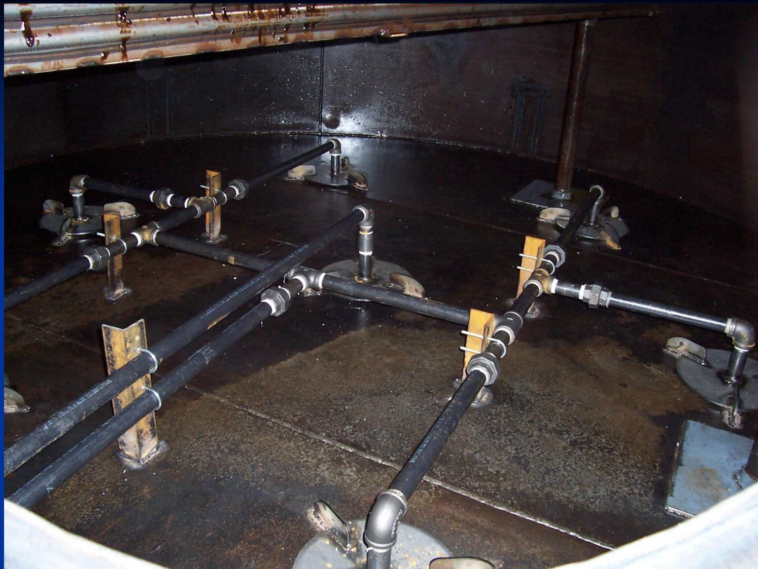
Carbon steel plates & piping on the floor of a 10ft diameter lube blending tank.
