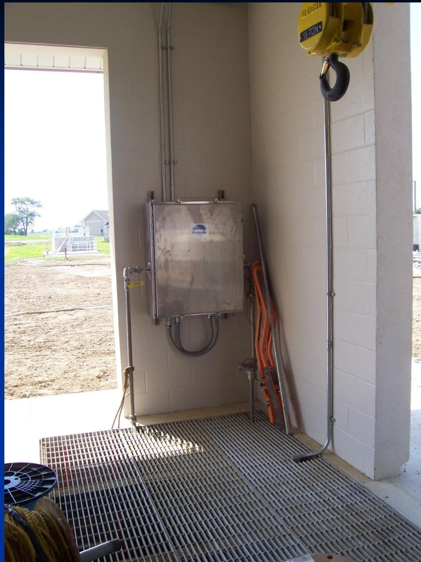
Pulsed Air system for mixing a lift station
