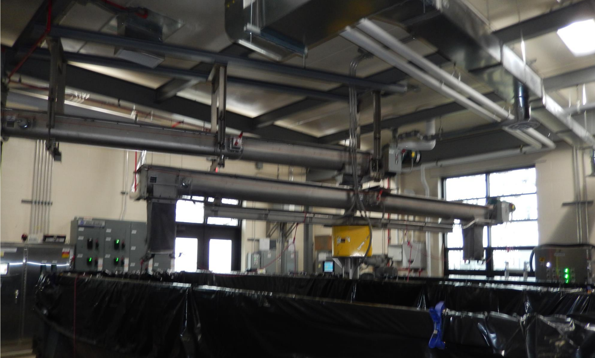
Gravity effects from elevated equipment
