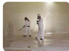
Figure 2c. Application of the chemical cleaning agent to remove organic and inorganic deposits on interior surfaces.
