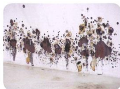
Figure 2b. Locations where the interior coatings had failed in the Ryan Ranch tank (these were repaired).
