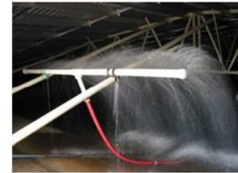
Figure 2: Aeration at Denmark Horsley Road Reservoir
