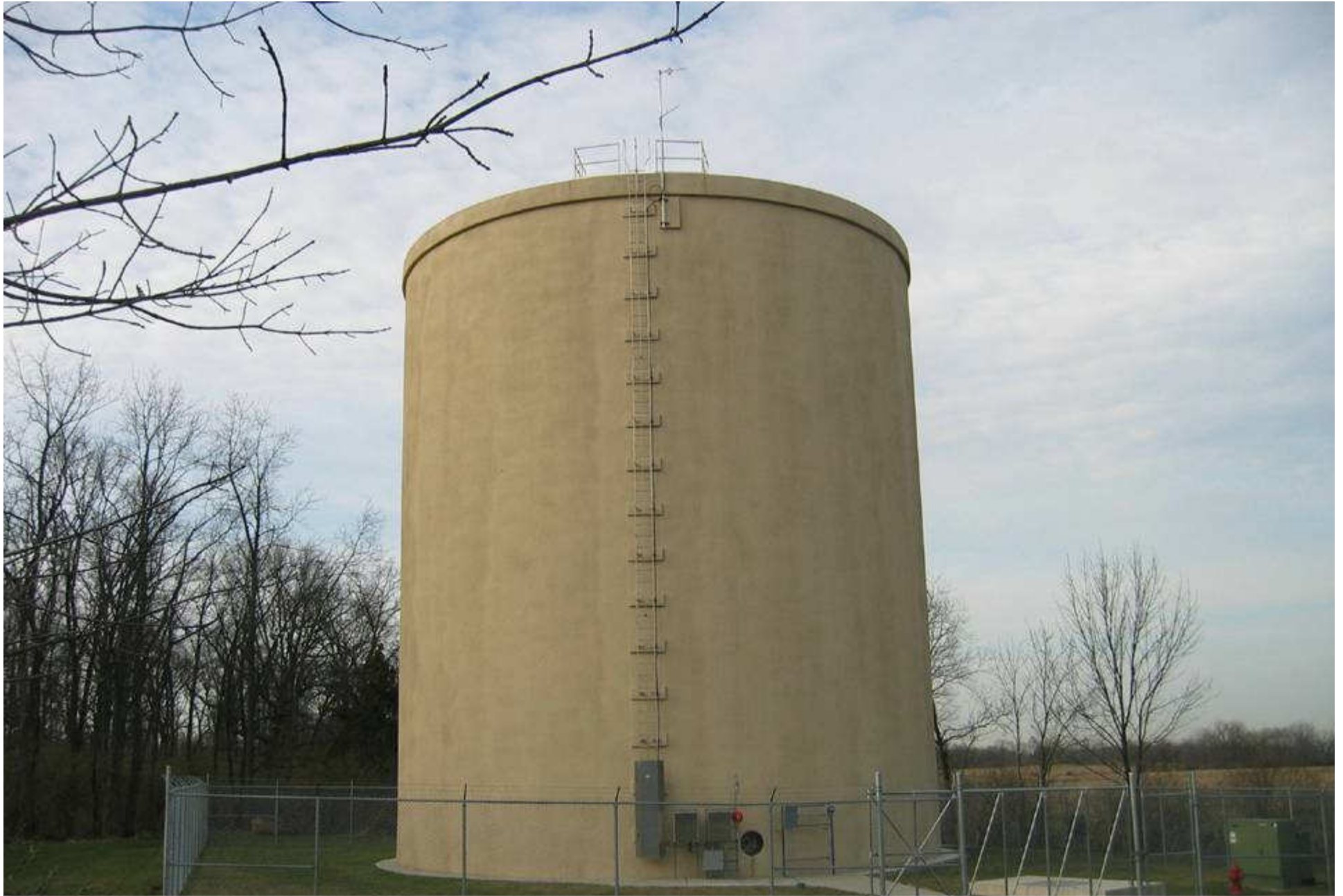
Enon, OH (Springfield) Water Storage Tank 1.0 MG 53' diam x 61' swd Owner: Clark County Utilities Engr: Lockwood, Jones & Beals
