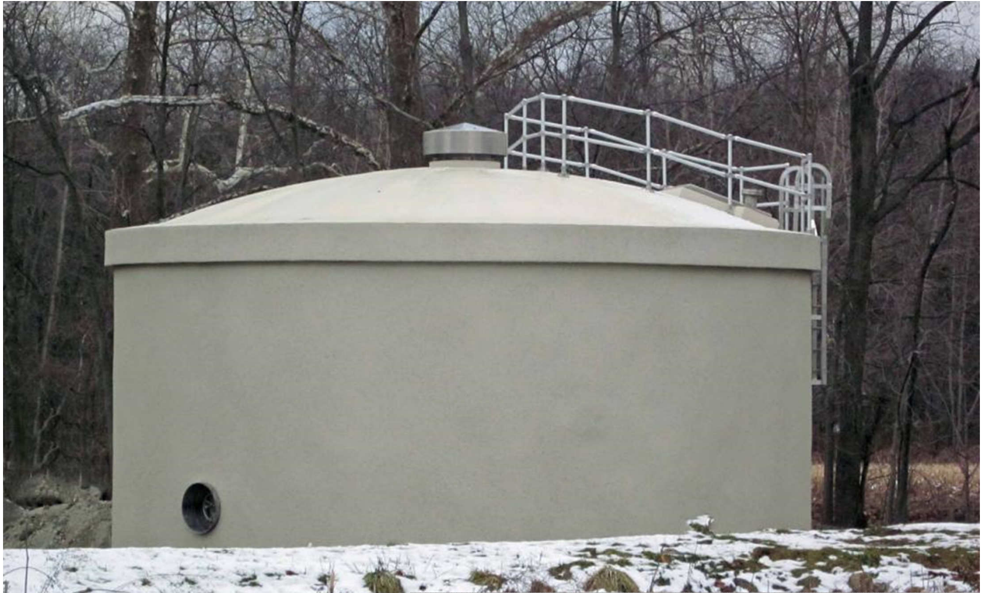
Pierceton, IN 2011 86,000-Gallons, 30' Diam x 16.5' SWD Owner: Town of Pierceton Engr: GRW Engineers
