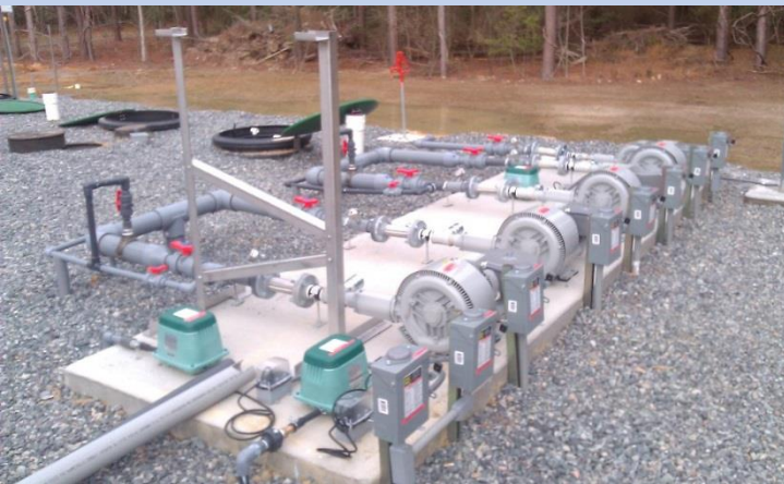
Regenerative Blower (multi-train installation)
