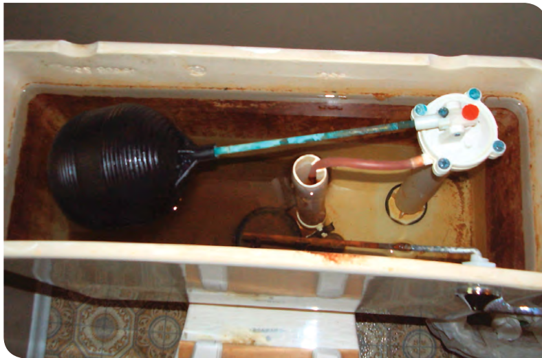
Figure 7-1, Slime Build-up in Toilet Tank
