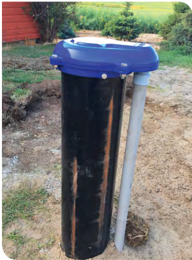
Figure 3-10, Installed Vermin-Proof Well Cap
