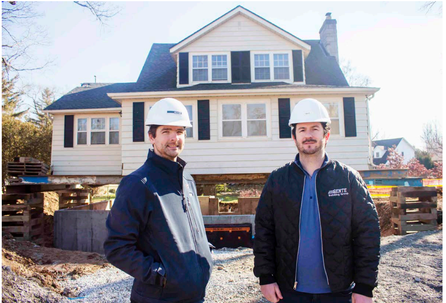
Tom Janzen, left, and Matt Hozack look forward to seeing the house at 10 Circle St. lowered onto its new foundation.. EVAN LOREE
