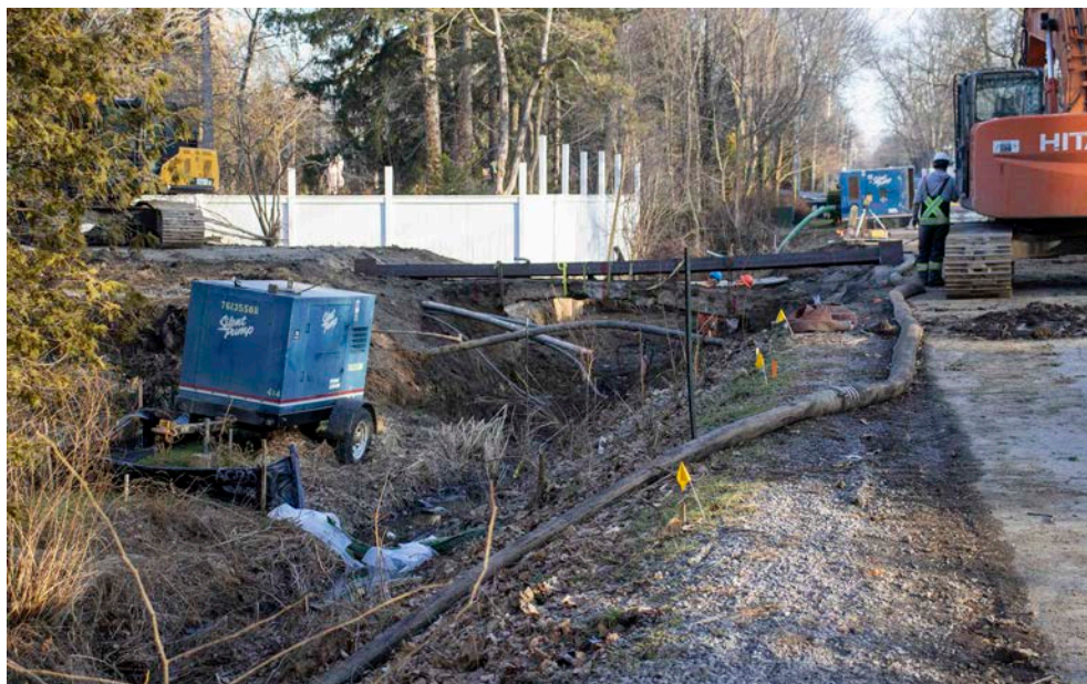
Construction of the new culvert at Johnson and Simcoe Streets continues, despite concerns that the historic old stone culvert would be destroyed. The town intends to save as much of the stone as possible for use in other town projects. SOMER SLOBODIAN
