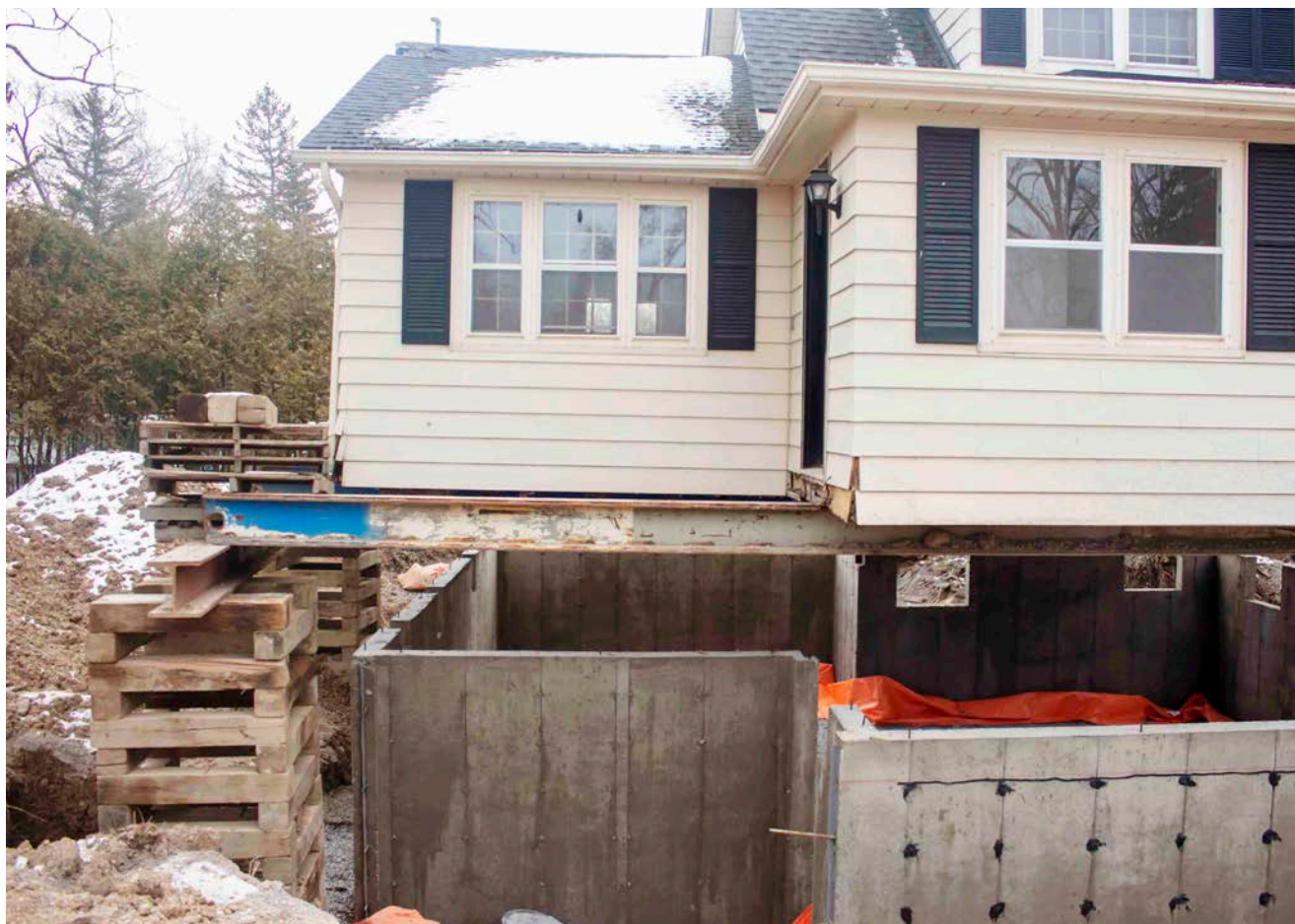
It took the team five hours to raise the house to put in a new basement. EVAN LOREE
