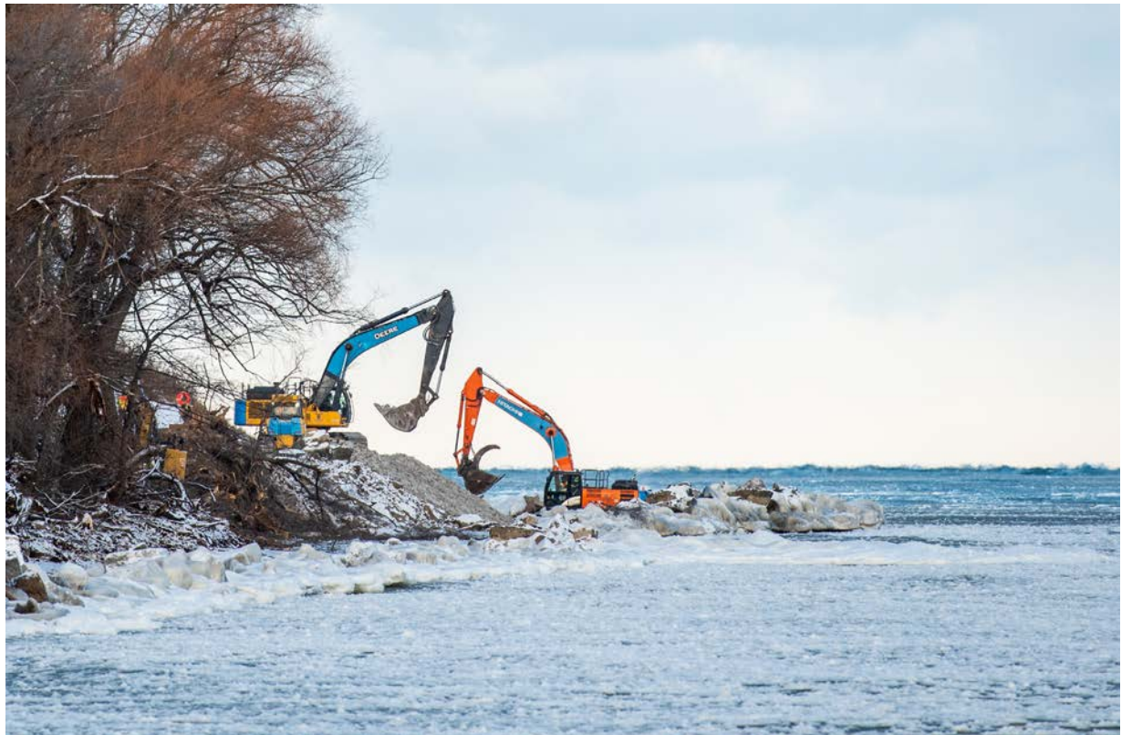
Work to protect the Lake Ontario shoreline from erosion is underway at Fort Mississauga. DAVE VAN DE LAAR
